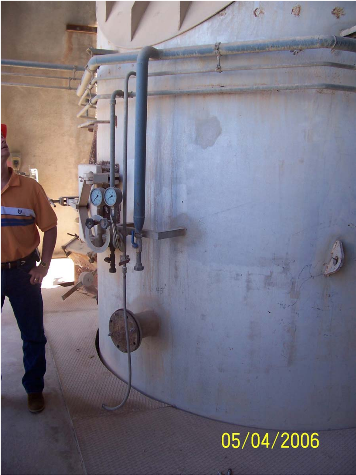
FIGURE 5 Disconnected SCR ammonia injection system
