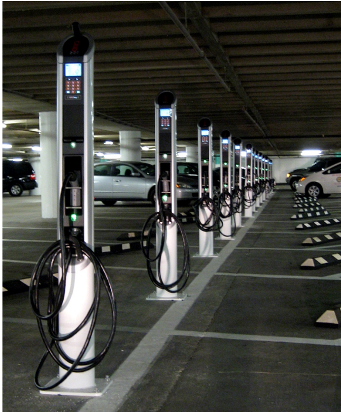
Figure 1: Phase 1 Installation at the City of Houston Tranquility Parking Garage
