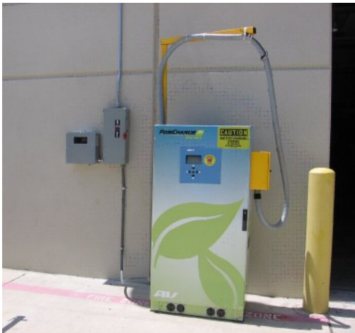
Figure 1. Proterra bus charger installed at Capital Metro facilities.
