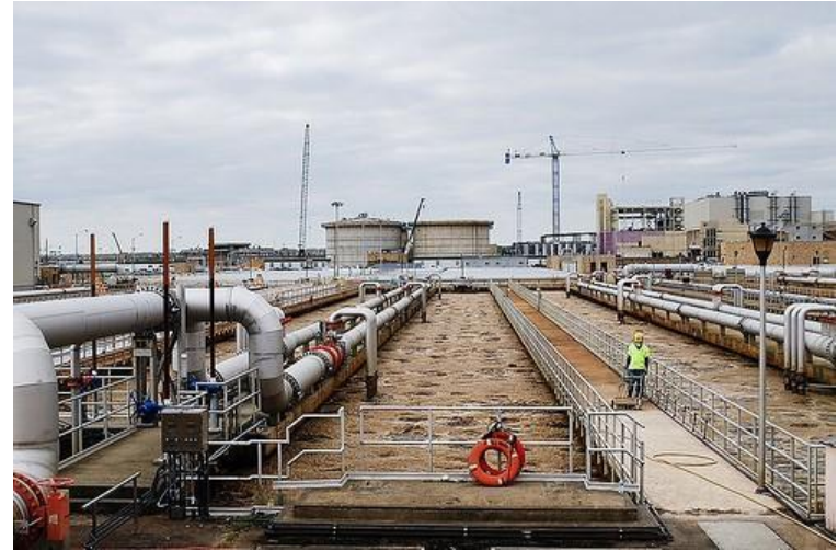
Wastewater Treatment Plant
