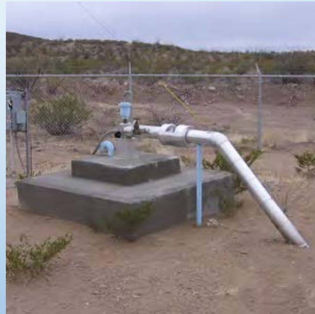
Example source water location: well head
