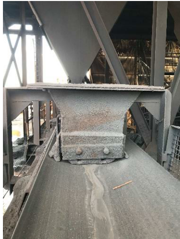
Figure 4.4.2.1 – BC22 Transfer Point at TT21
