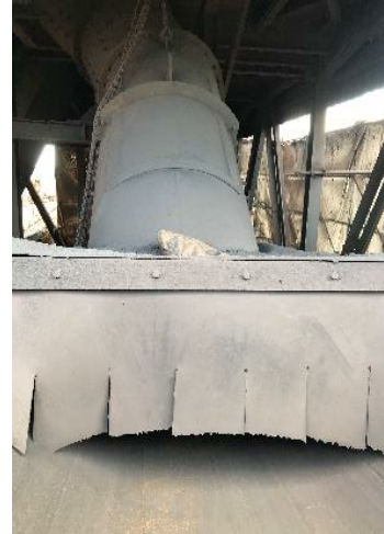
Figure 4.4.2.1 – BC23 Transfer Point at TT21
