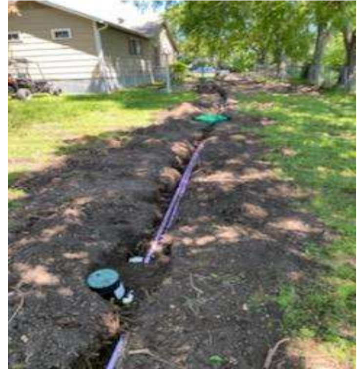
Texas RC&D replaced a non-functional septic system for a resident in Collin County, Texas (SEP No. 2012-07)
