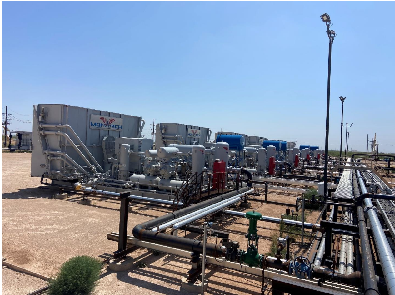
Figure 5- View of all Compressors installed
