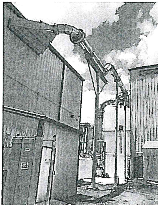
Figure 4. Photographs of the supplementary ductwork, dampers, and valves.
