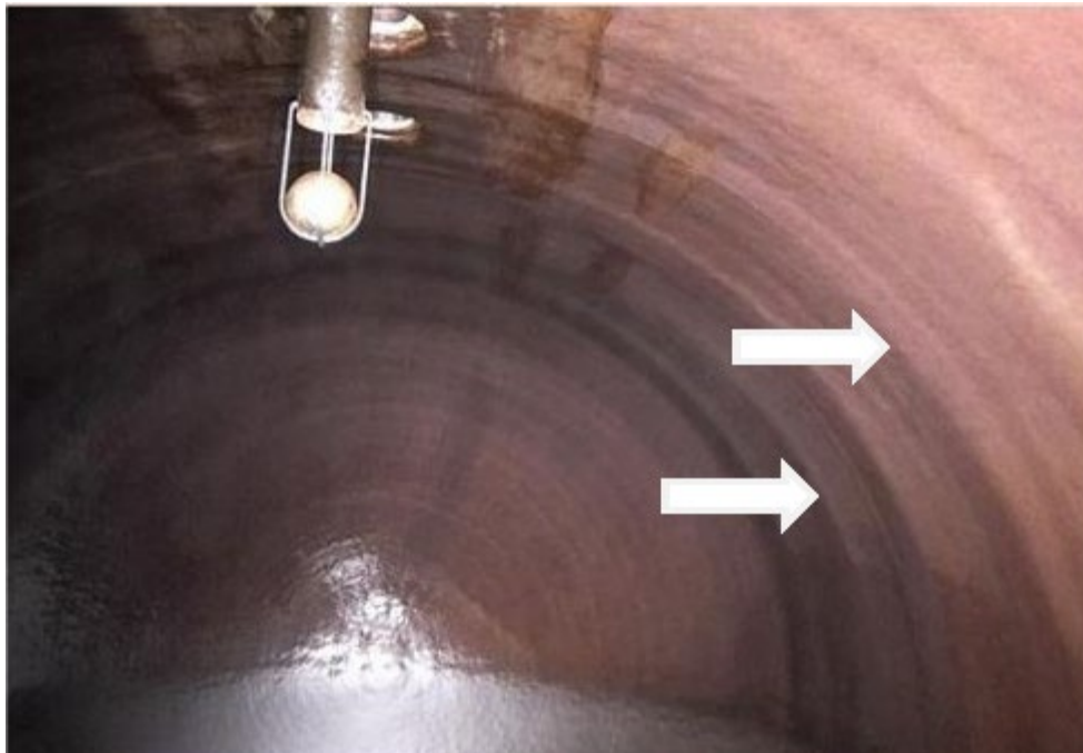
Figure 5. FRP Tank "Ribs" Seen Through Internal Camera Survey
