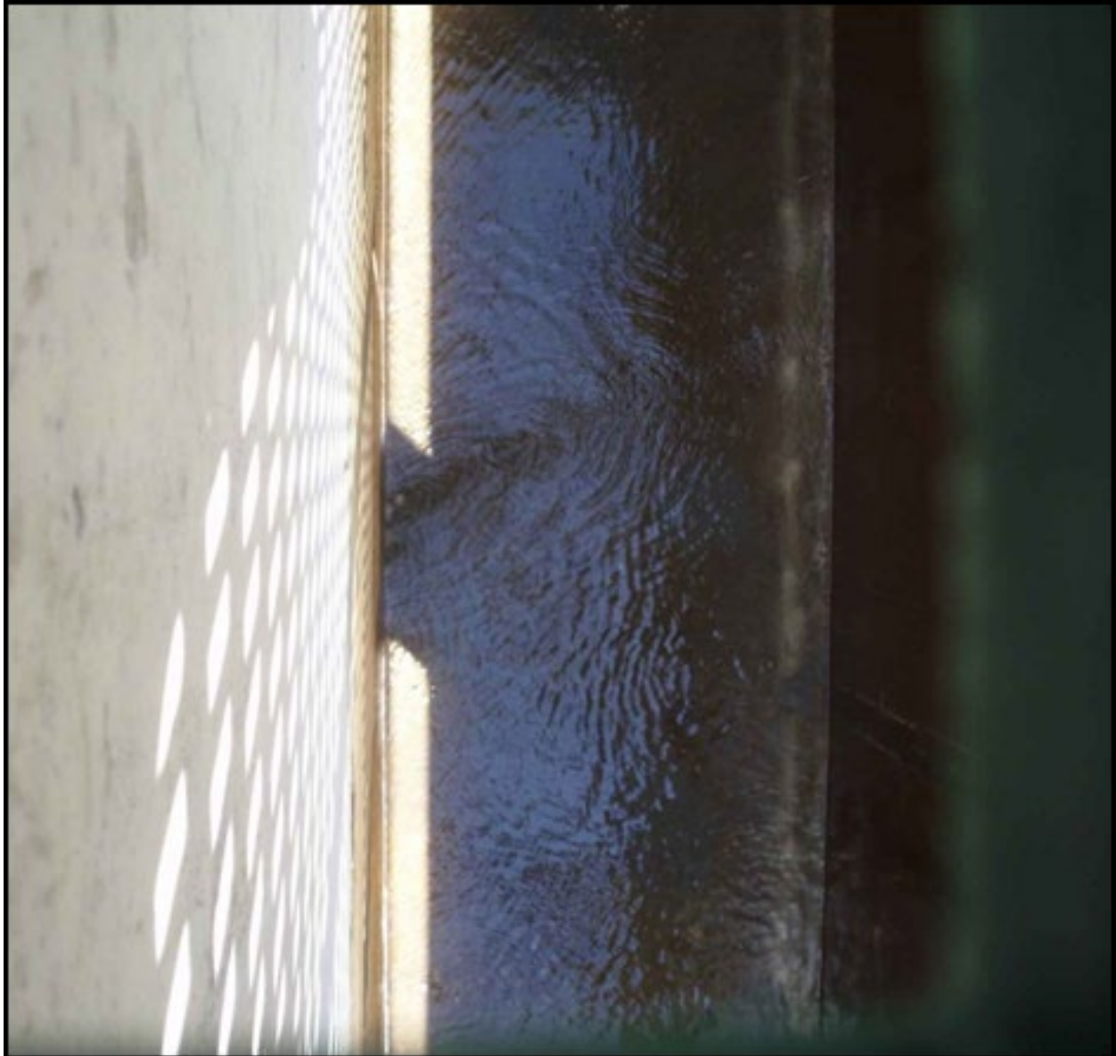
Figure 44: Filter Box Cross Connection
