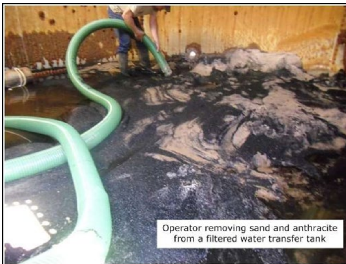
Figure 29: Filtered Water Transfer Tank with Sand and Anthracite
