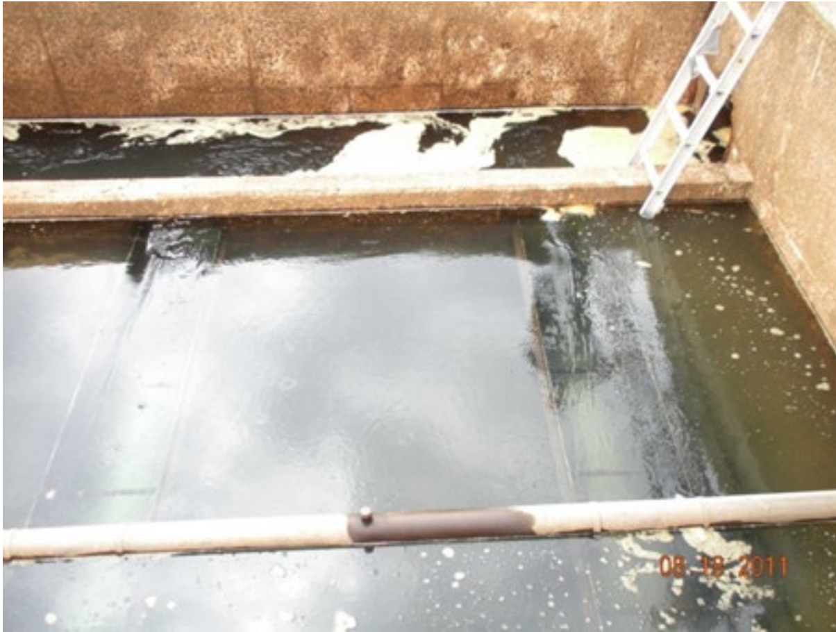
Figure 37: Examples of Trough Flooding
