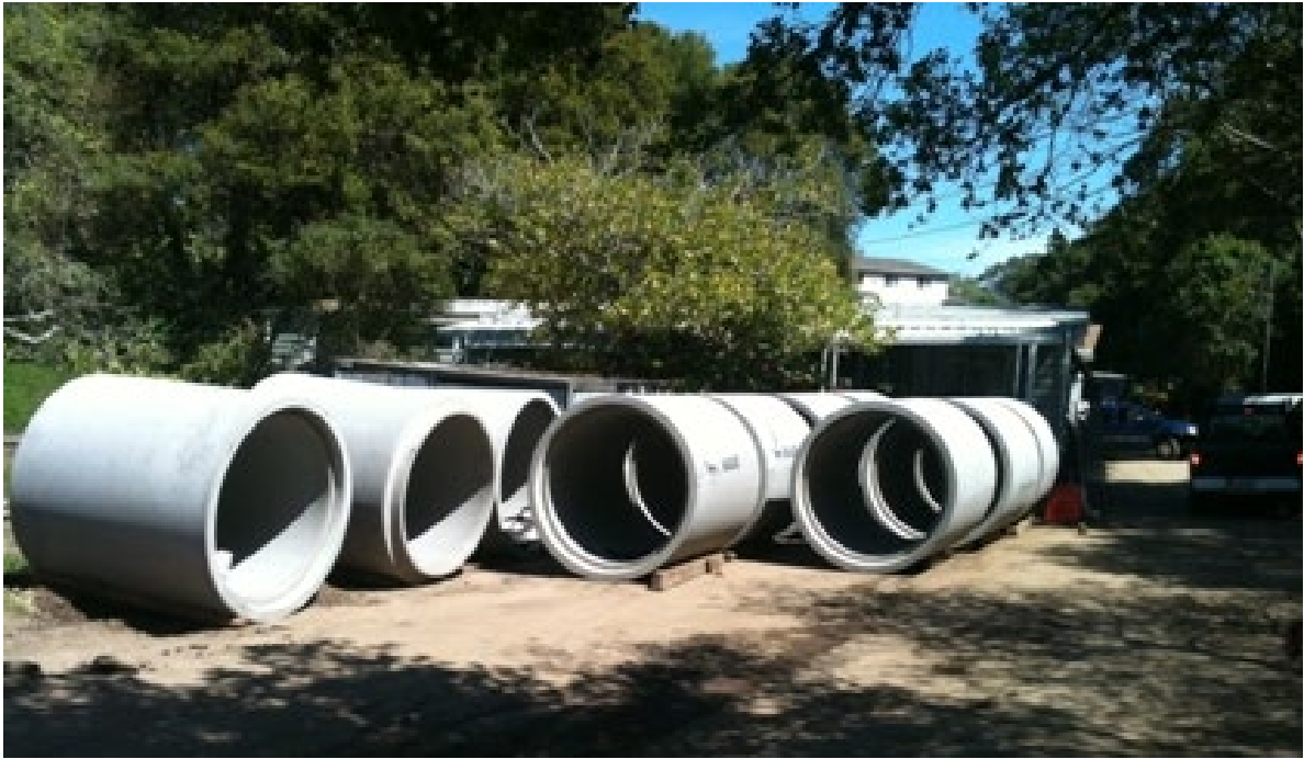
Figure 14. When pipes are stored outside, they are vulnerable to contamination
