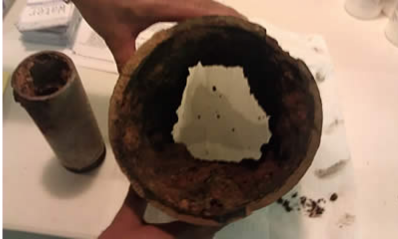
Tubercular plating in an iron pipe
