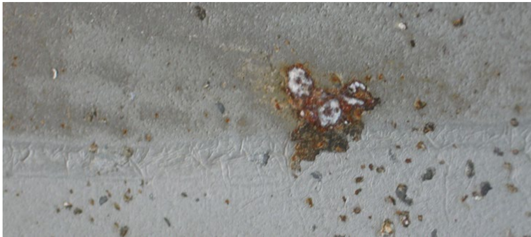
Figure 24. Pin-hole corrosion on a steel tank
