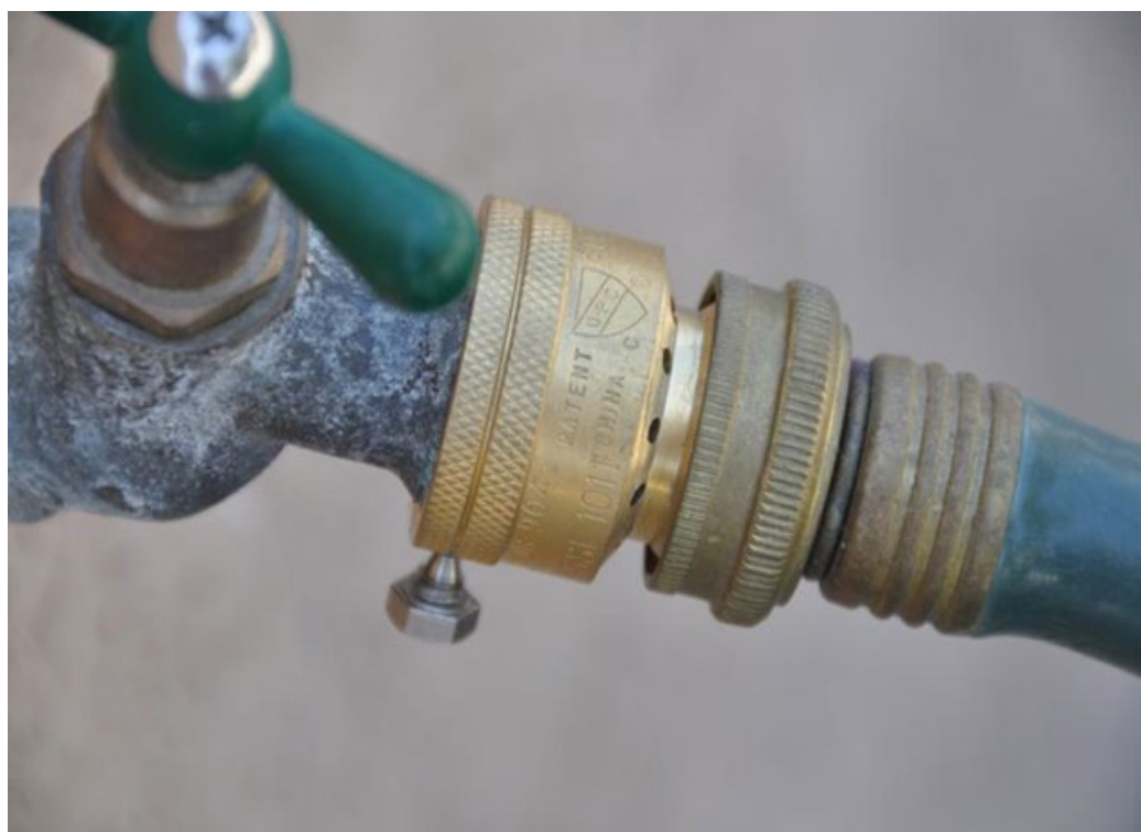
Figure 31: Photograph of a hose-bibb vacuum breaker.
