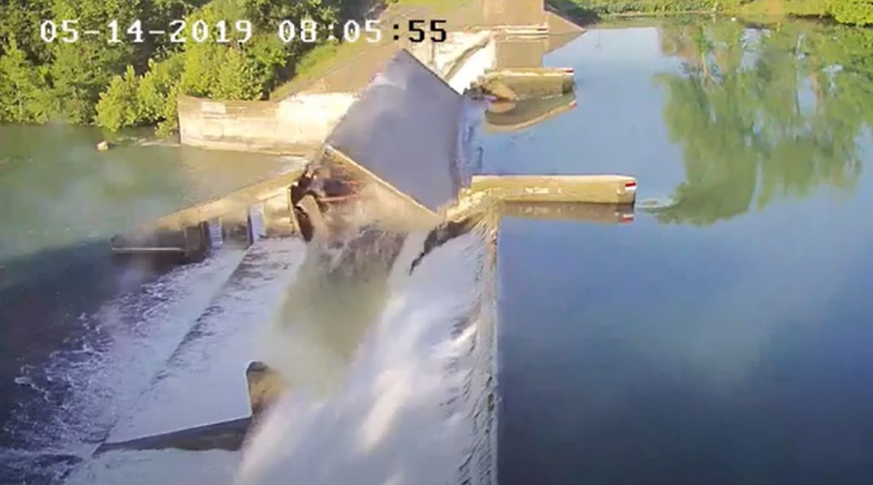
Lake Dunlap Dam Spillway Failure
