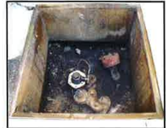
Uncontained turbine sump
