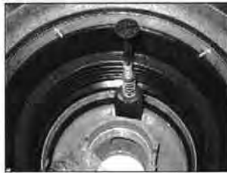
Spill bucket drain valve
