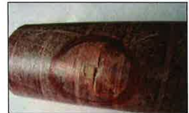
Fiberglass piping is cracked
