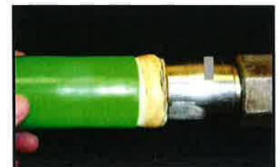
Flexible piping is bulging
