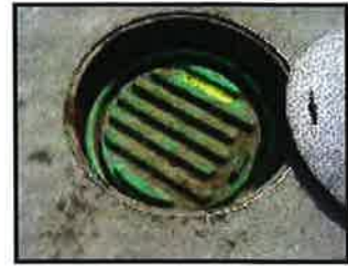
Circular steel sump lid pulled back to show the inner lid covering the turbine sump
