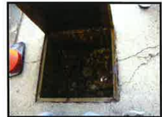
Square steel sump lid pulled up to show the inside of an uncontained turbine sump
