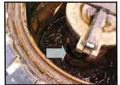
Spill bucket in poor condition – note the gap between the spill bucket and the fill pipe
