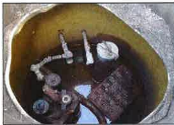
Contained sump with liquid and debris
