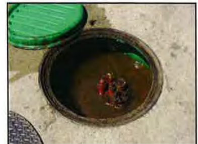
Contained turbine sump full of liquid
