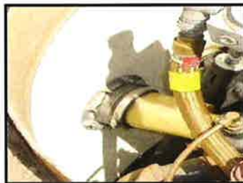
Sump penetration seals in good condition
