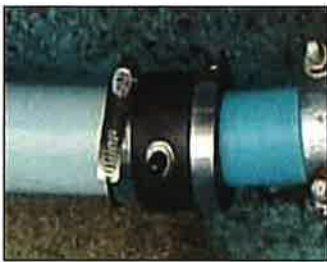
Test boot located in a sump
