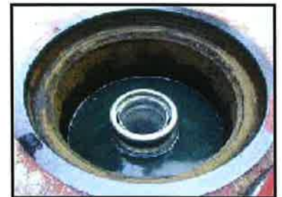
Spill bucket that contains liquid
