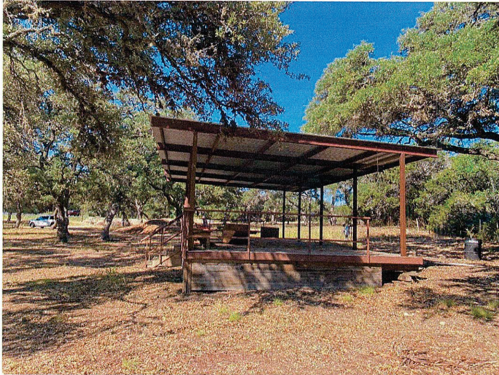
Photograph 8: West facing view of ground obstruction.
