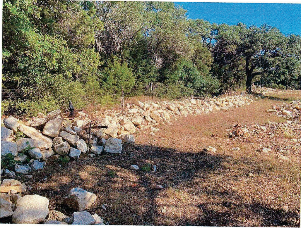
Photograph 4: North facing view of ground obstruction.
