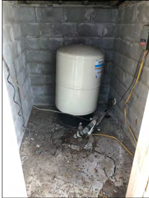
3 - View of well head and pressure tank
