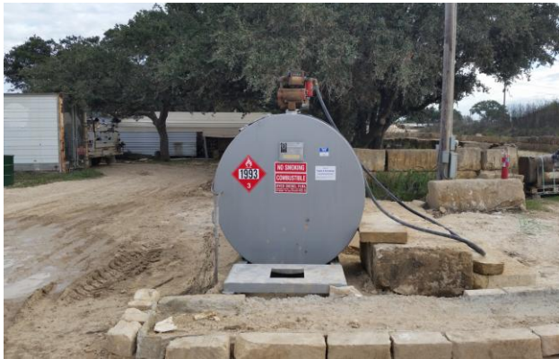
19. Front view of 3,000-gallon diesel fuel double-walled AST located just to the west of the maintenance area.
