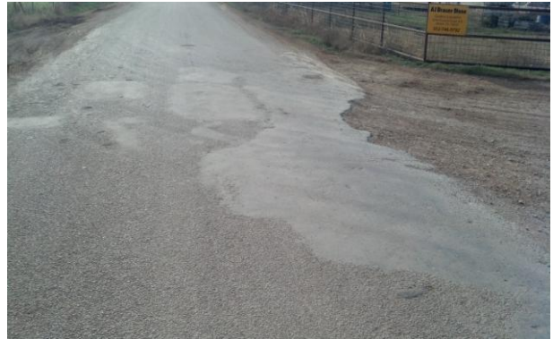
10. View of surface of CR305 at northern quarry entrance/exit. Note very little material is tracked from the property onto CR305.
