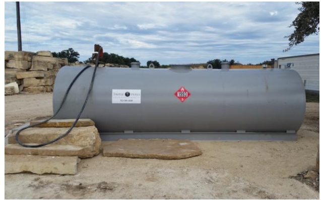
18. Side view of 3,000-gallon diesel fuel double-walled AST located just to the west of the maintenance area.
