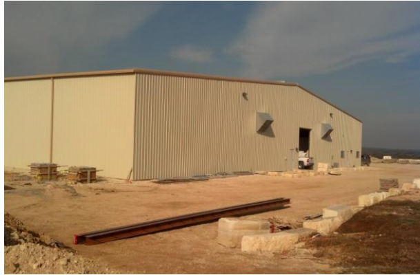
1. View of fabrication building located on southeast portion of AJ Brauer Stone property. This building is covered by a previously TCEQ-approved WPAP.
