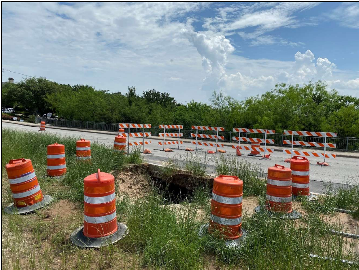
Feature Photo MPS-33 Non-karst Closed Depression (Photo 1 of 3). Traffic barriers were in place surrounding the hazard. Photo taken on April 8, 2020.
