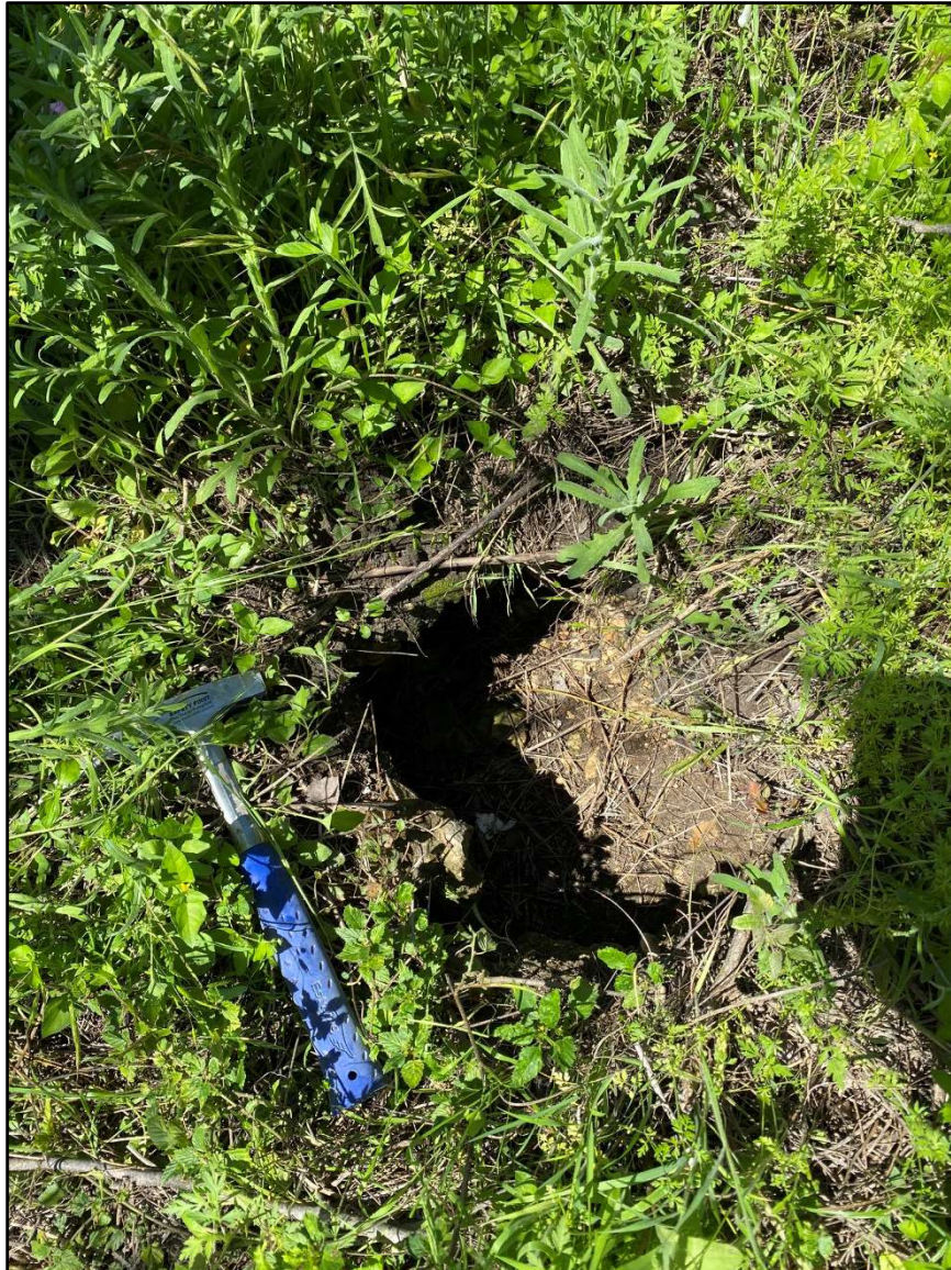
Feature Photo MPS-30 Non-karst Closed Depression. This closed depression is likely related to the existing utility line. No bedrock exposures are present.
