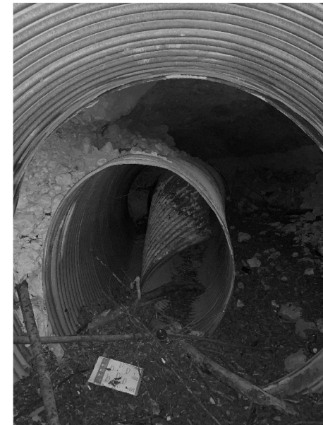
PHOTO OF COLLAPSED CMP IN VOID AREA
