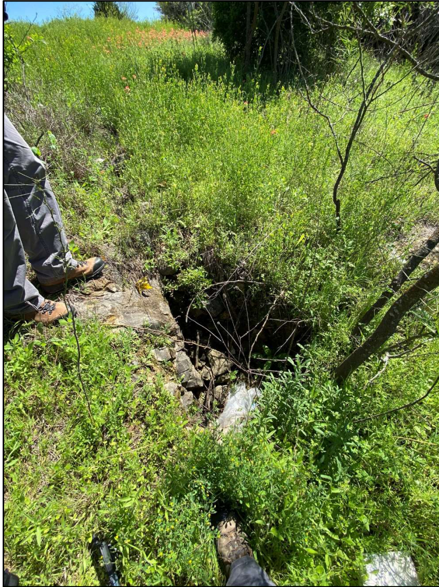
Feature Photo MPS-31 Non-karst Closed Depression. This closed depression is likely related to the existing utility line. No bedrock exposures are present within the depression.
