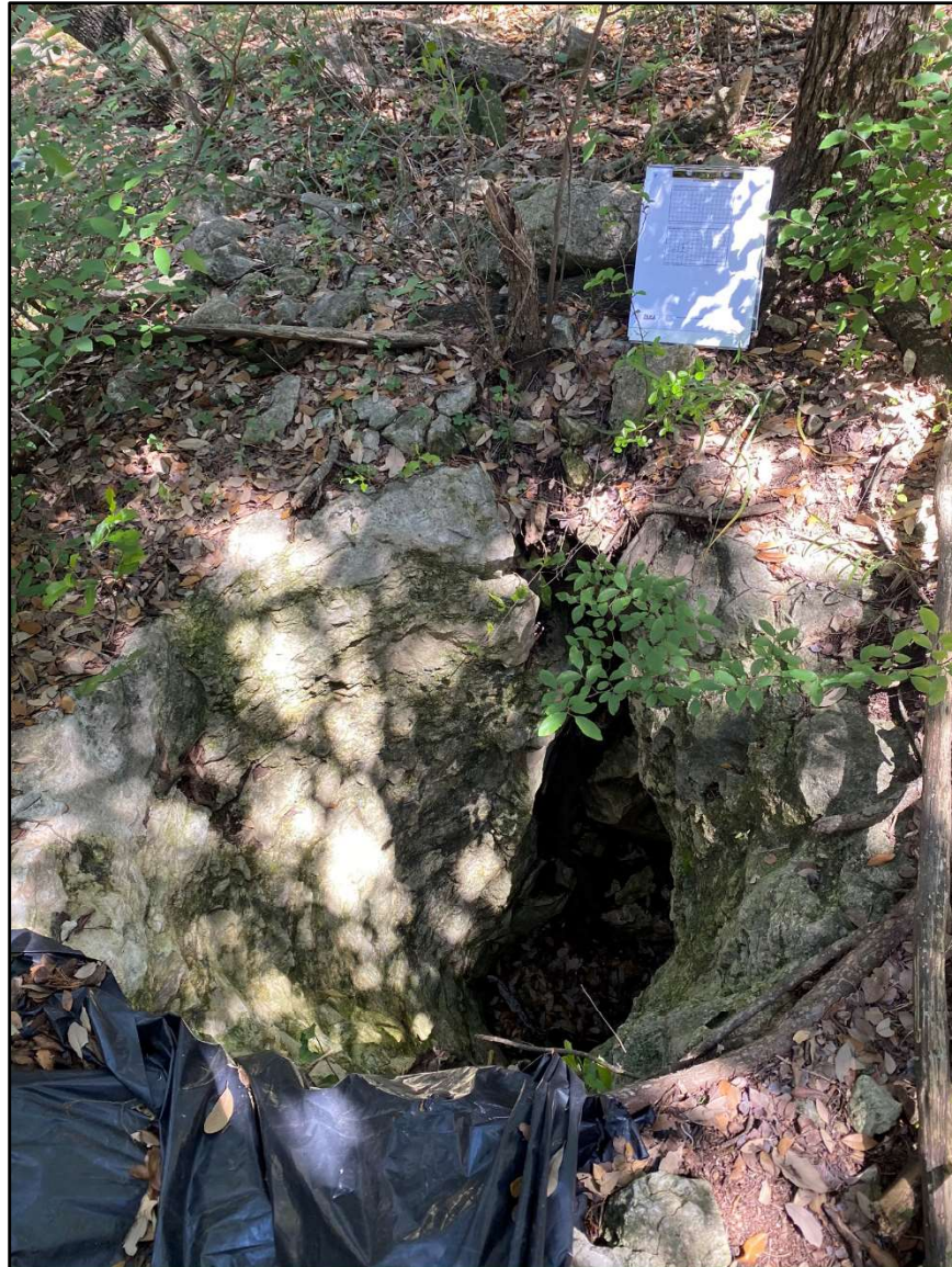
Feature Photo MPS-7 Solution Cavity. Remnant plastic tarp and plywood covers from a previous investigation are present near the opening.
