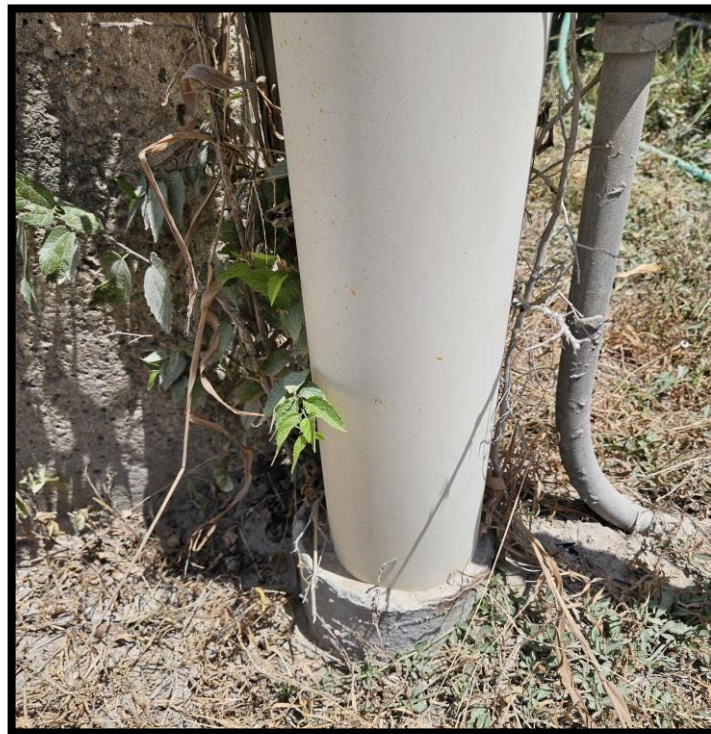
S-1: PVC casing and steel surface sleeve showing no evidence of damage or erosion.
