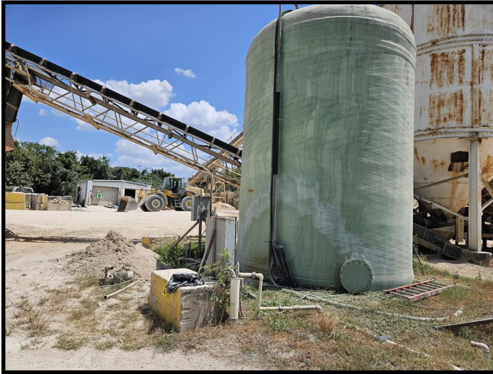
S-1: Water well view from the north.
