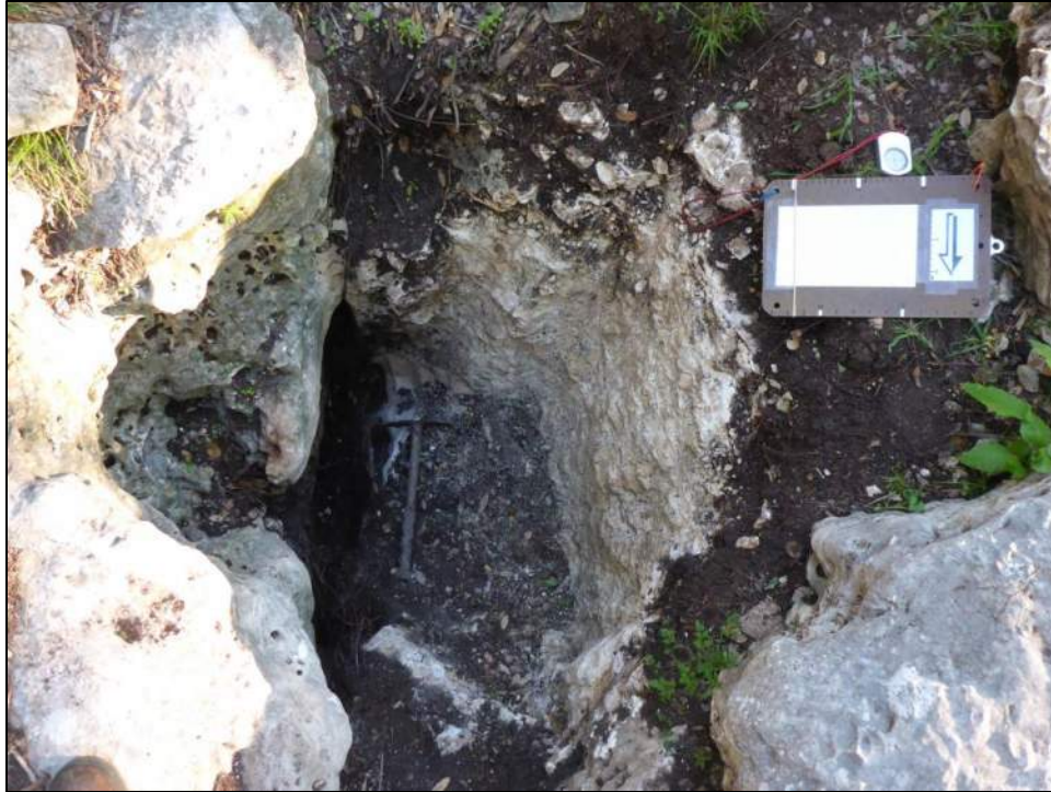
Figure 36. Feature AV12/X7 after excavation. Note the soil filled fracture potentially continuing downward. The fracture narrows downward and further excavation was not justified.
