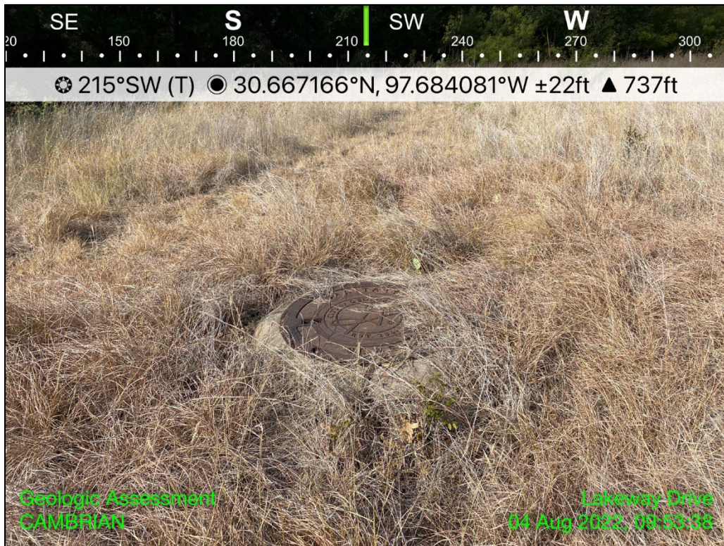
Photo 8. View of the existing wastewater utility on the property.
