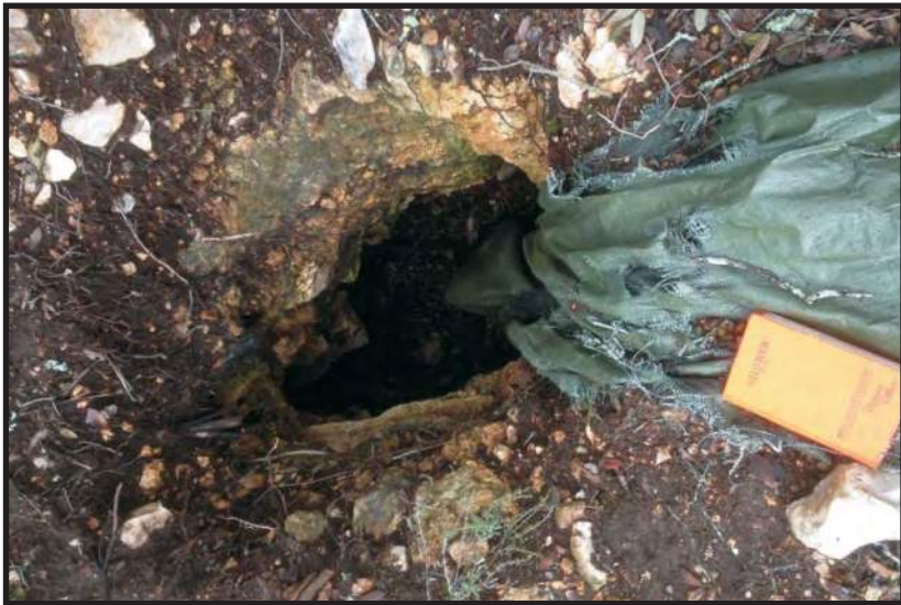
PHOTO 51 Close up view of geologic feature F-33 (NF-5, solution cavity)
