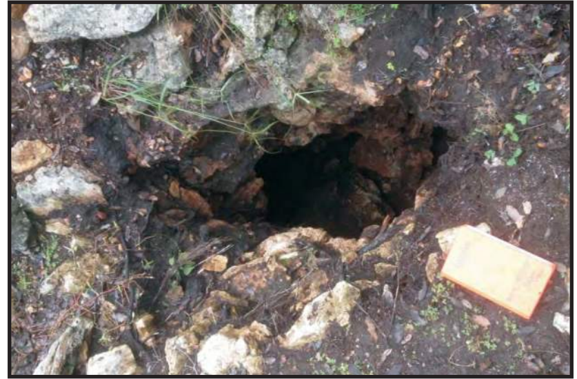
PHOTO 50 Close up view of geologic feature F-32 (NF-7, solution cavity)
