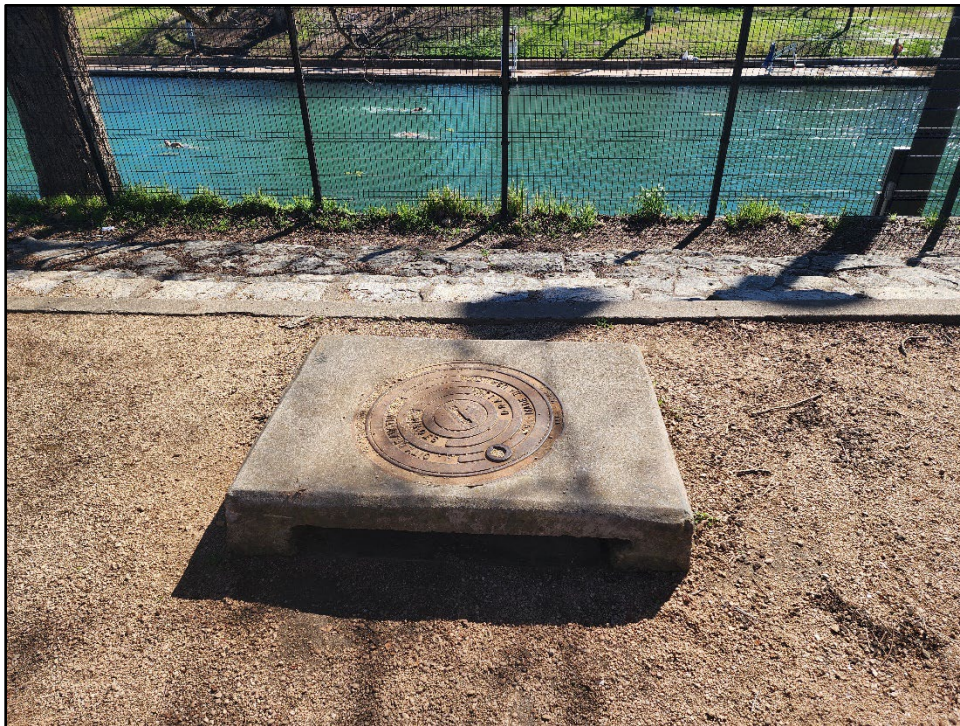
Figure 9. Example of stormwater infrastructure associated with MB-04.
