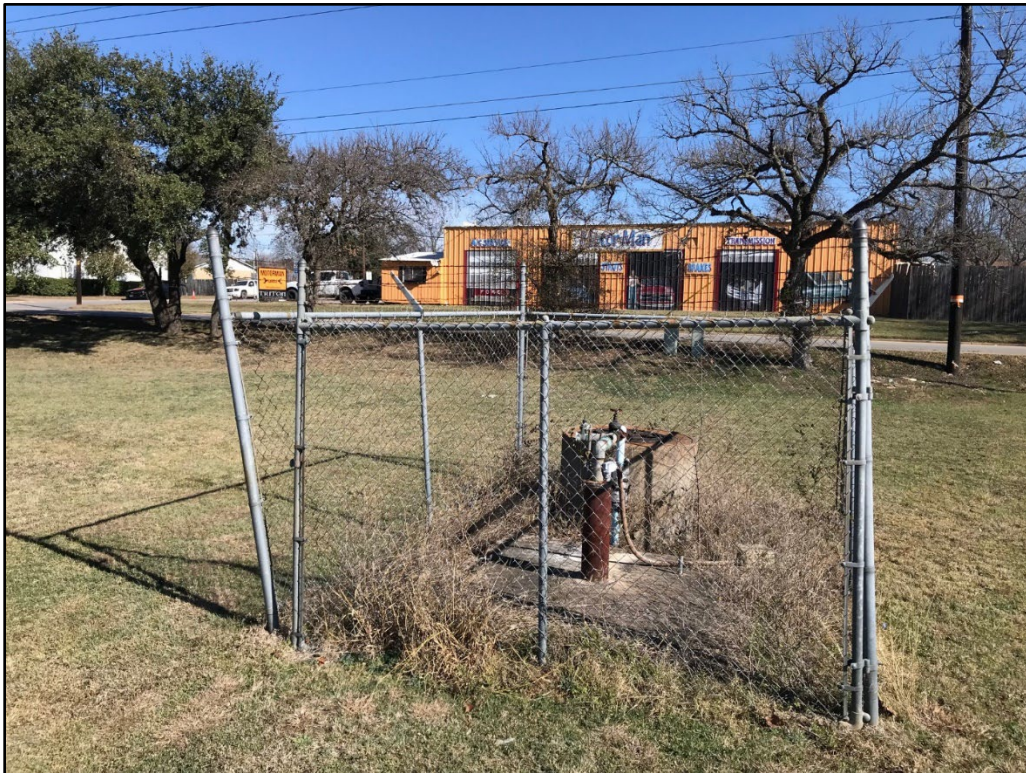
Photo 4. Water well W-1 is protected within a fenced enclosure.
