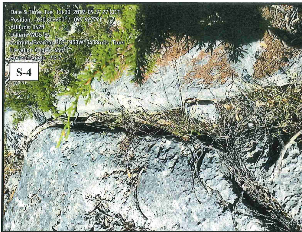
S-4 Solution-enlarged fracture just inside the northern fence line.
