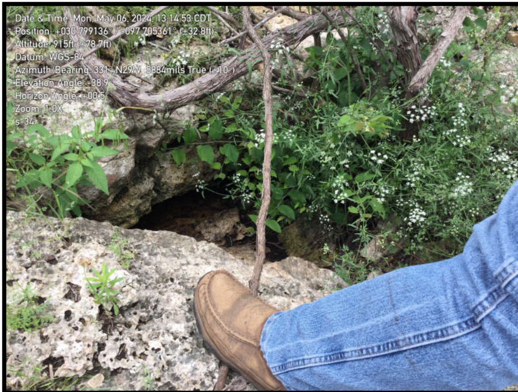
S-34: Solution cavity located within a sinkhole.
