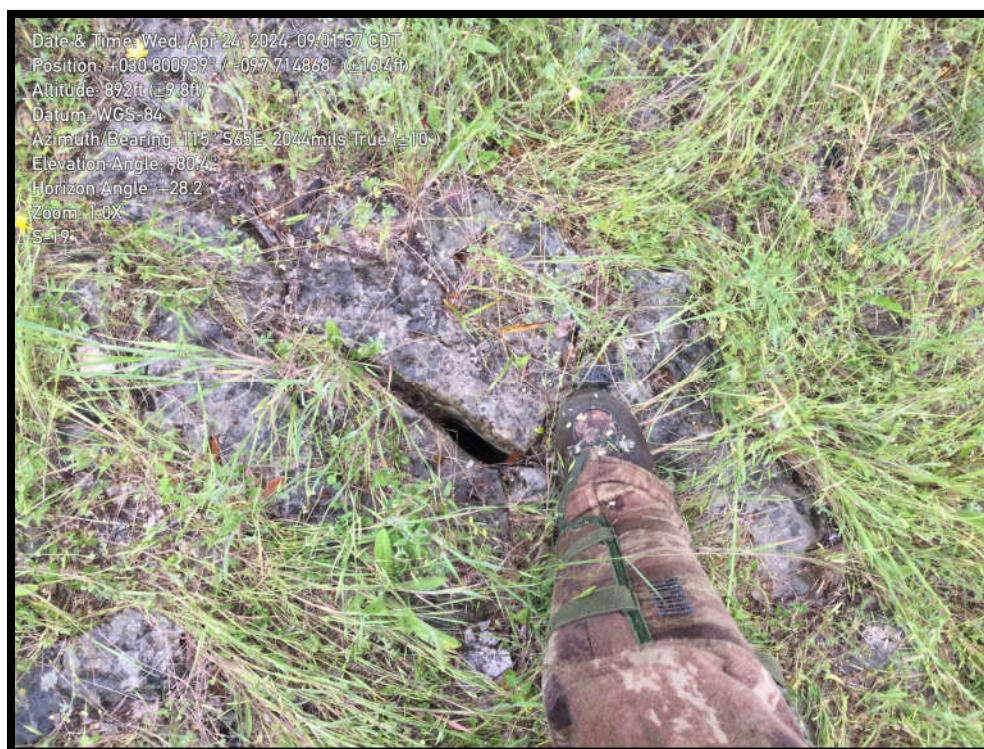
S-19: Solution-enlarged fracture located on the northwestern part of the Site.
