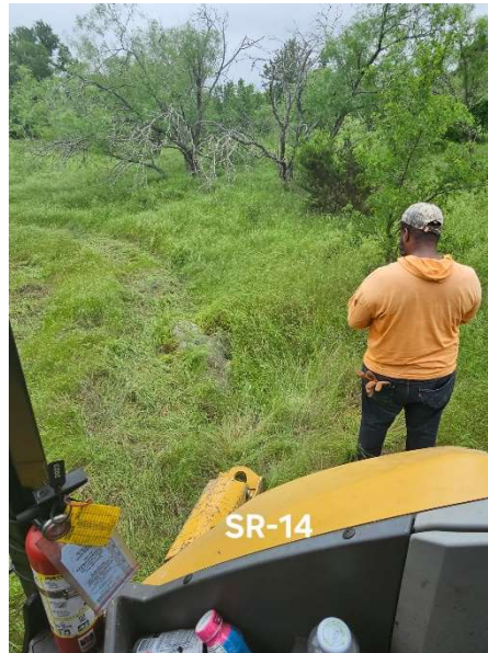
Geologic feature SR-14 (sinkhole) before excavation, facing south
