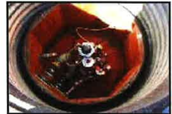
Contained turbine sump
