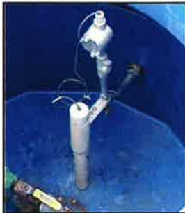
Float sump sensor
