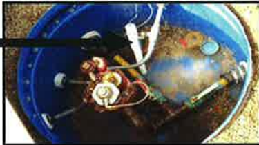
Sump sensor in contained turbine sump
