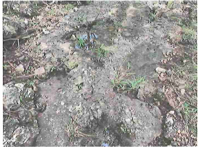
Ponding Water on Vuggy Limestone in Dry Drainage Feature
