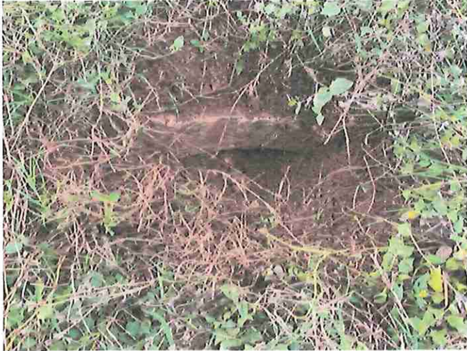
CD-1 – Non-Karst Closed Depression within Manmade Berm
