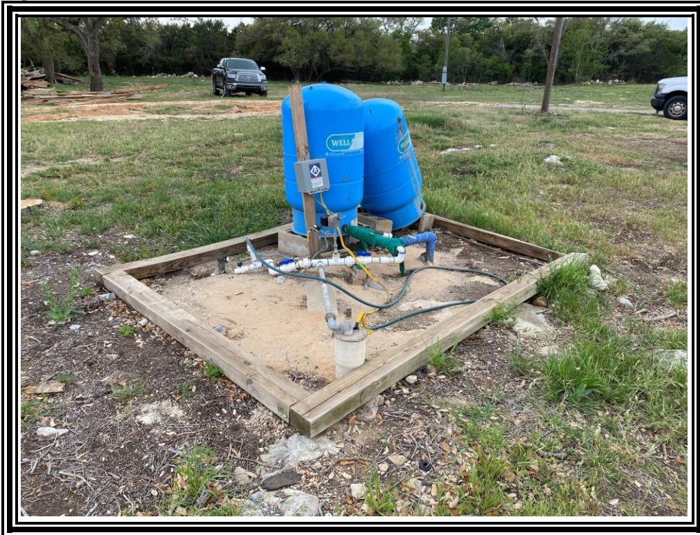
5. View of water well feature S-1, in the north-central portion of the site.
