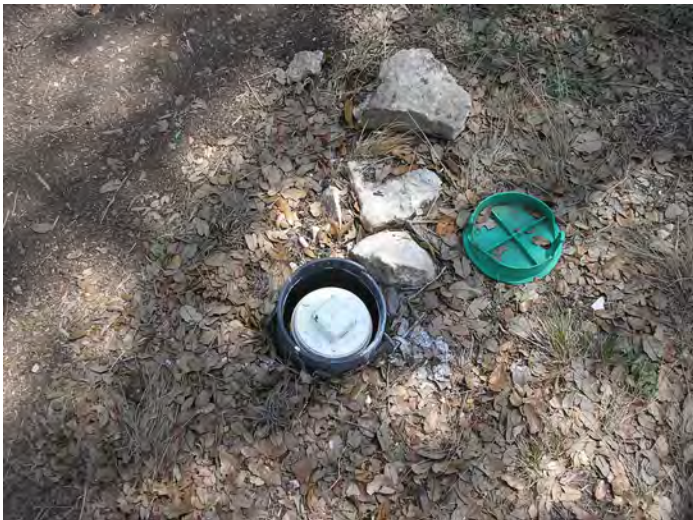
Photo #19 – View of PRF #S-11. A suspect septic system.
