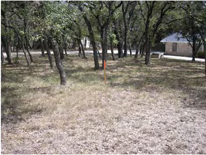
Photo #25 – View of an additional survey stake marking the location of a proposed sanitary sewer manhole.
