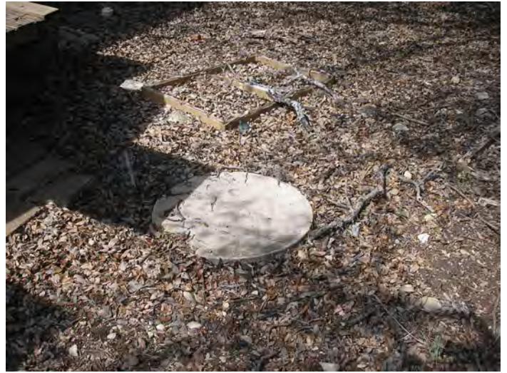
Photo #10 – View of PRF #S-6. A suspect septic system.
