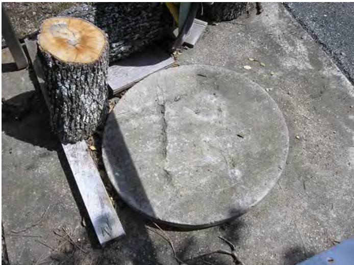
Photo #11 – View of PRF #S-7. A suspect septic system.
