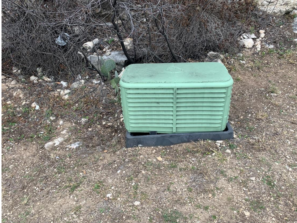
Photo #10: View of telecommunication box at the location of feature S-5. Photo taken January 6, 2023.
