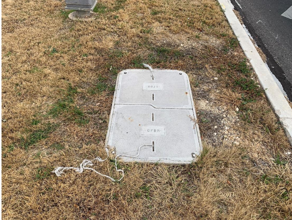
Photo #8: View of Google Fiber communication manway box at the location of feature S-3. Photo taken January 6, 2023.
