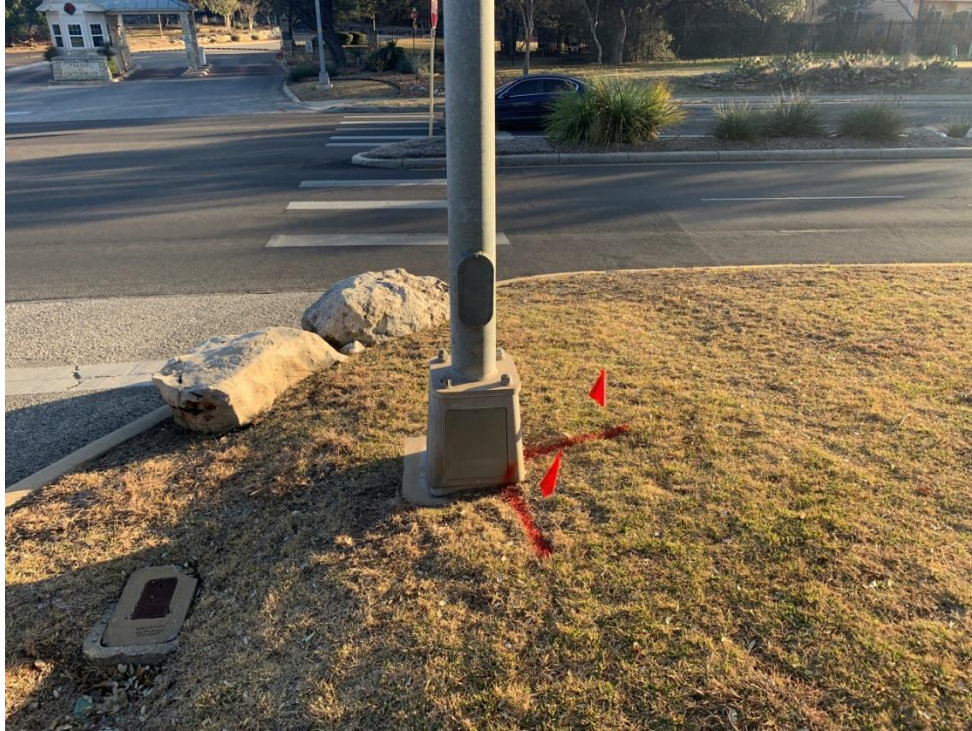
Photo #13: View of traffic light post and marked electric line at the location of feature S-11. Photo taken January 6, 2023.
