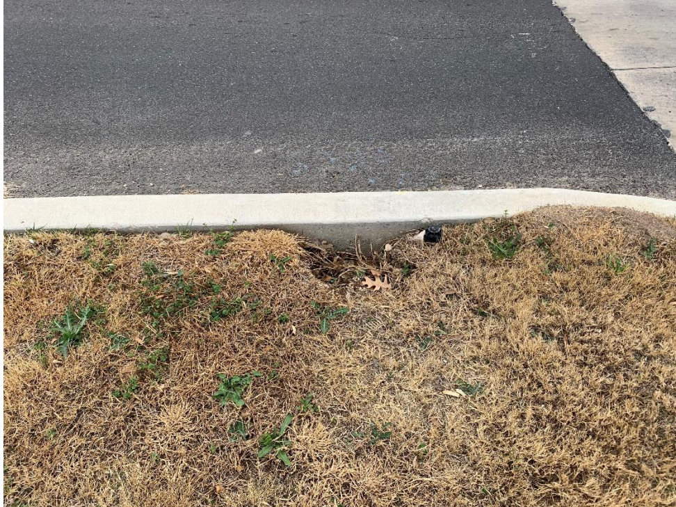
Photo #6: View of excavated soil and rotor head sprinkler at the location of feature S-2. Photo taken January 6, 2023.
