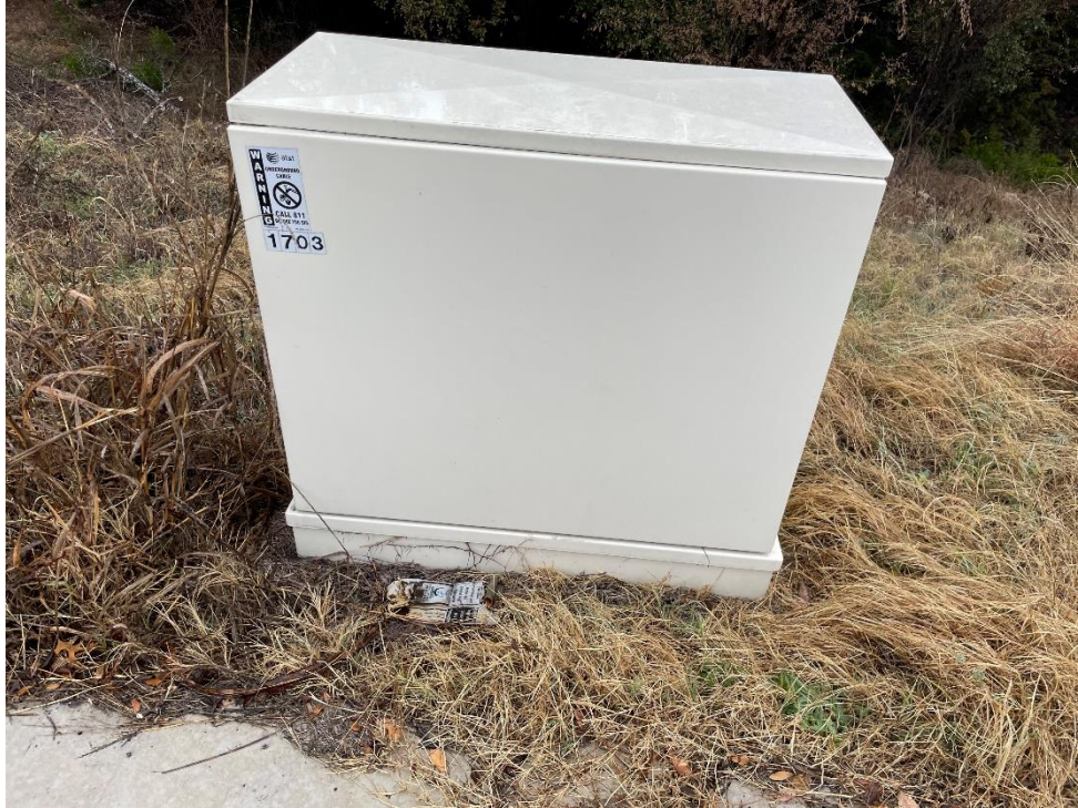
Photo #13: View of AT&T utility box at the location of feature of feature S-10. Photo taken January 28, 2023.
