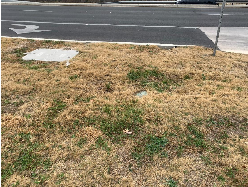
Photo #5: View of suspected irrigation manways and sprinkler head at the location of feature S-2. Photo taken January 6, 2023.
