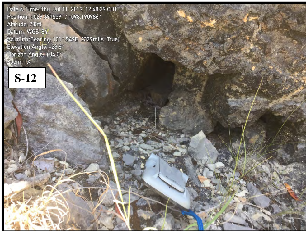
Feature S-12: Solution Cavity at the base of a historic highwall
