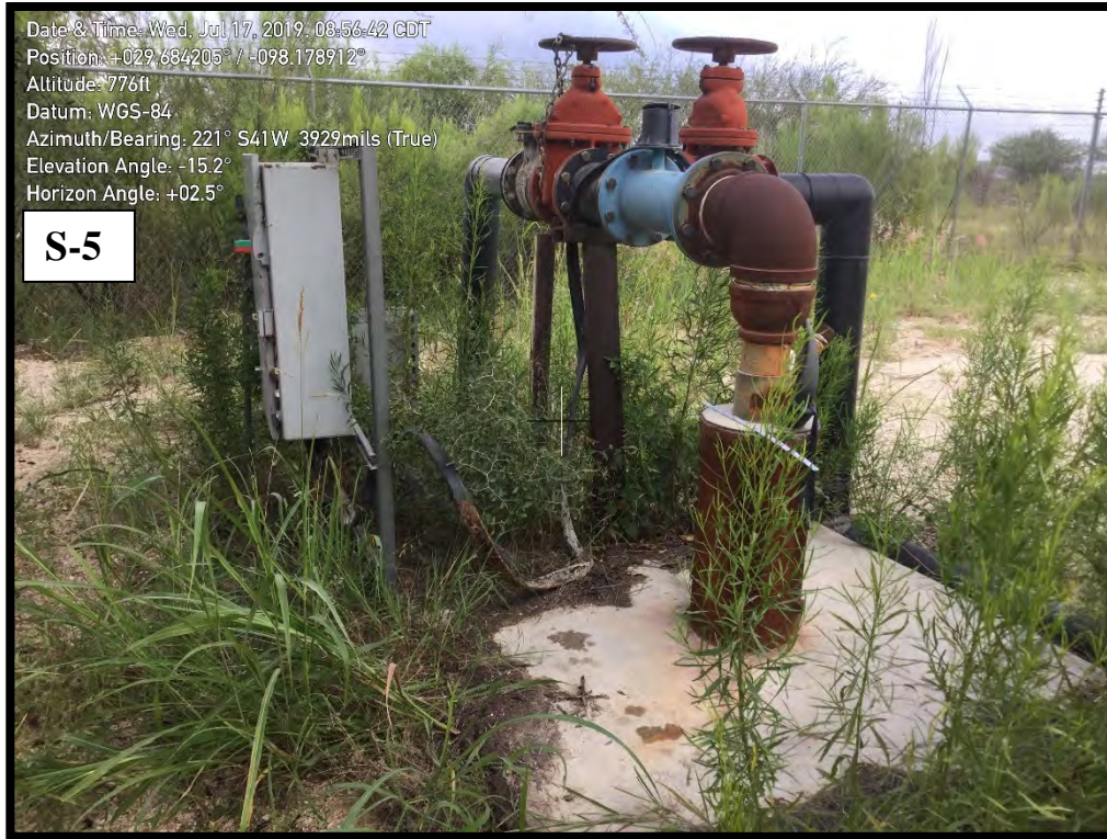
Industrial water well, S-5, on the northwestern part of the Site.
