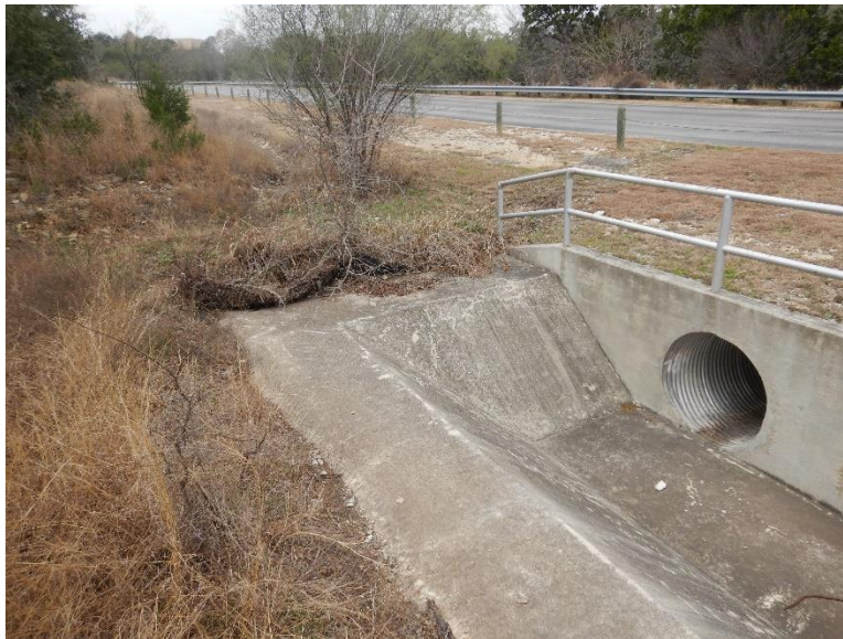
Photo 3. View looking west along Gold Canyon Road from culvert at bedrock lined drainage swale.
