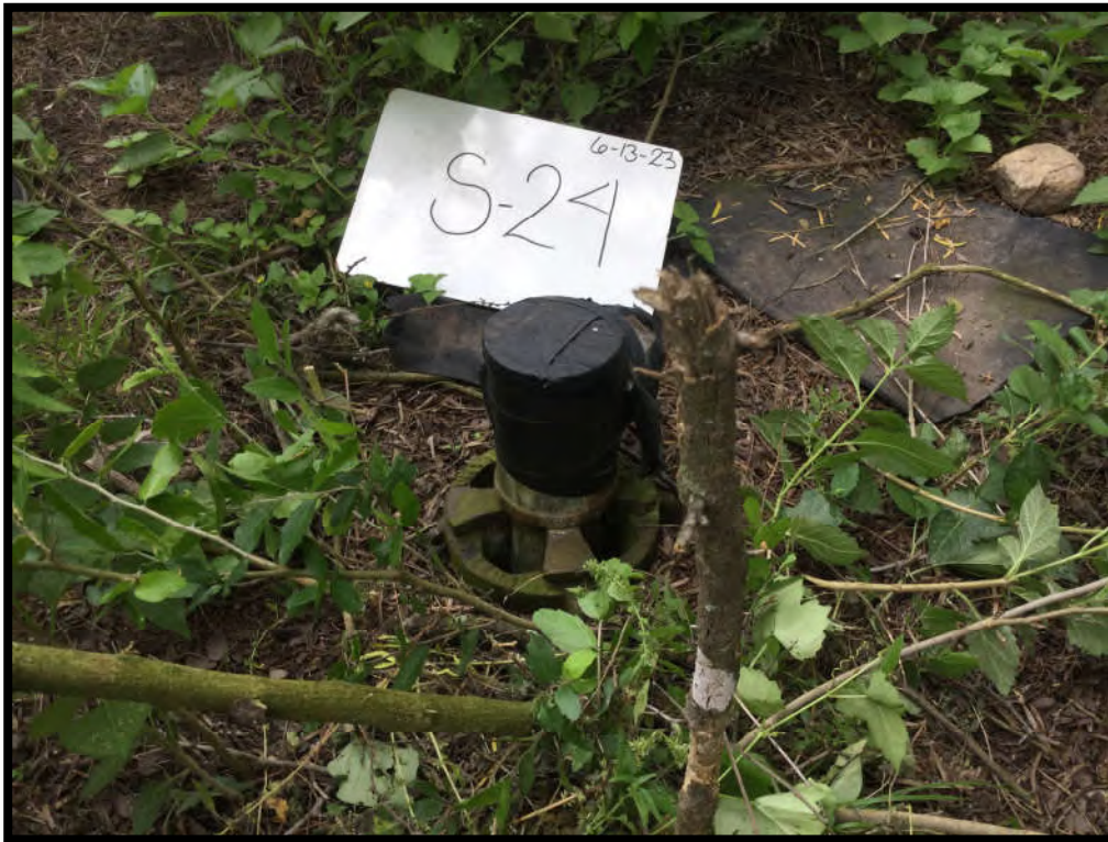
S-24: Water well historically powered by a windmill located on the southwest part of the Site.
