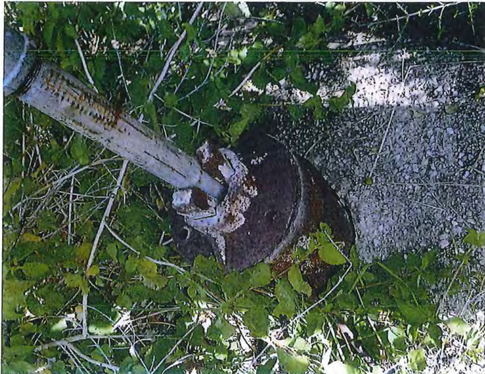
S-10: water well with separated casing, sensitive
