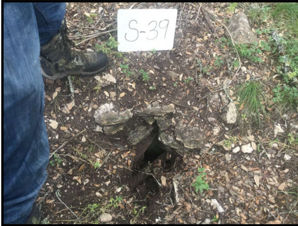
S-39: A solution cavity within the floodplain on the northwest part of the Site.
