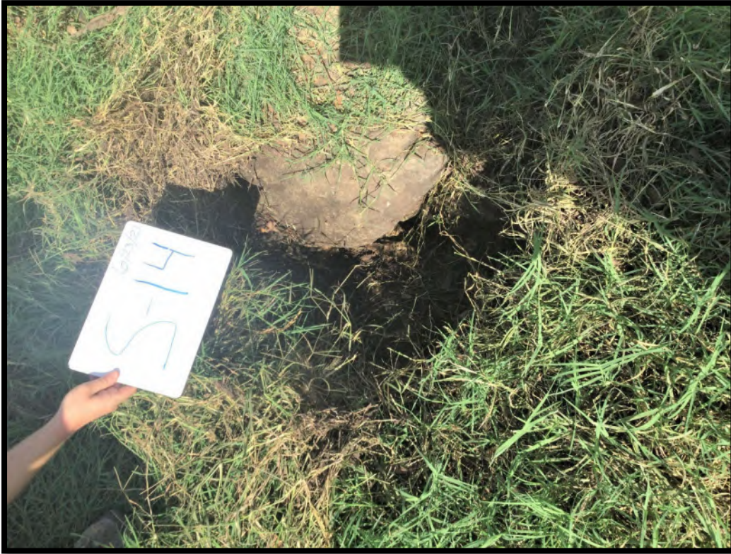
Feature S-14: Open solution cavity within the sensitive feature zone.
