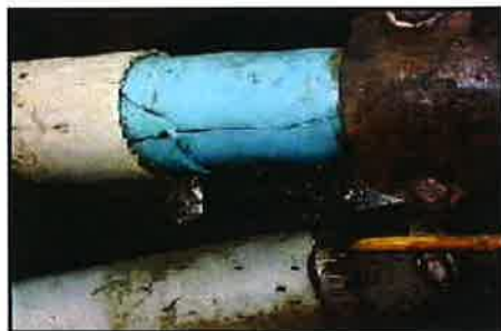
Flexible piping is cracked
