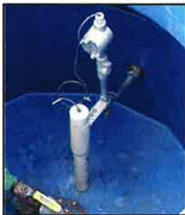
Float sump sensor
