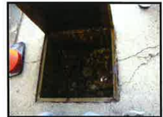
Square steel sump lid pulled up to show the inside of an uncontained turbine sump
