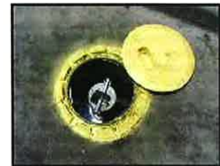
Circular spill bucket lid pulled back to show the fill port with a spill bucket
