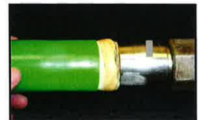
Flexible piping is bulging
