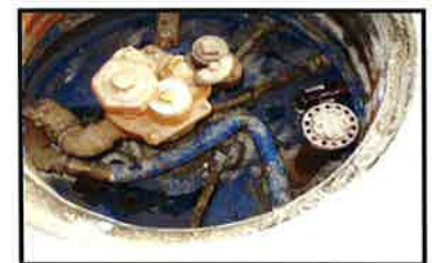
Flexible piping is kinked
