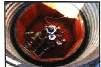
Contained turbine sump
