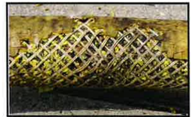
Flexible piping is degraded due to microbial growth
