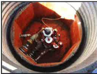
Dry, debris-free contained turbine sump
