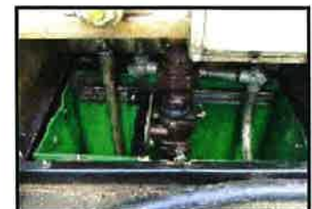
Contained dispenser sump
