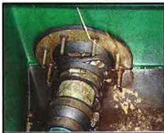
Sump penetration seals in poor condition
