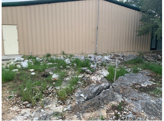
SF-1 Solution Enlarged Fracture
