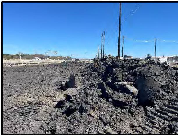
View toward the Culebra and Talley Road intersection of clay soils excavated along the north adjacent of project perimeter for the Culebra Road improvements.
