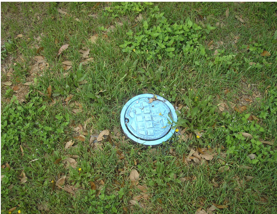
Photo #4: View of a marked 6-inch valve cover associated with feature S-2 in the vicinity of the east-central portion of the site immediately south of the intersection of Stonepath Drive and Crescent Oaks.
