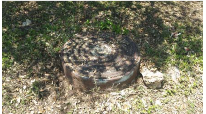
View of a Sanitary Sewer Manhole Cover, Potential Recharge Feature # S-4.
