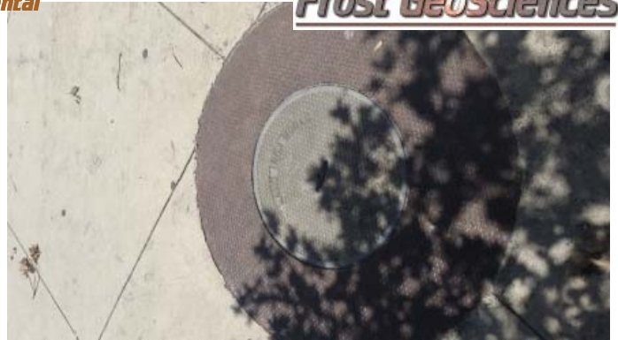
View of a Sanitary Sewer Manhole Cover, Potential Recharge Feature # S-2.
