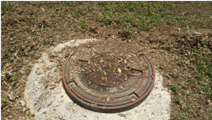
View of a Sanitary Sewer Manhole Cover, Potential Recharge Feature # S-3.
