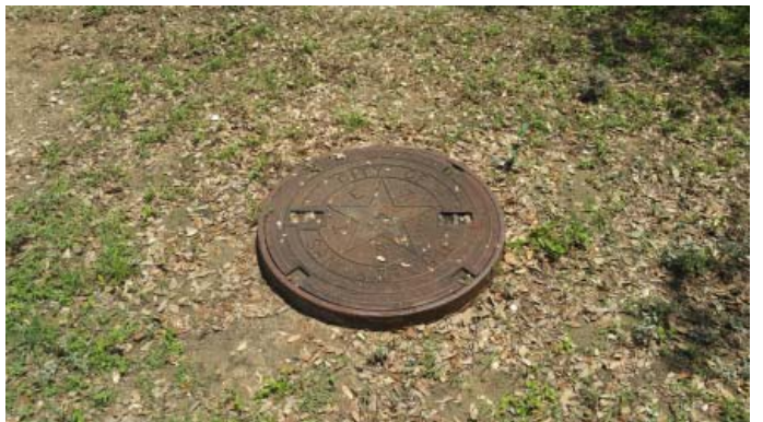
View of a Sanitary Sewer Manhole Cover, Potential Recharge Feature # S-6.
