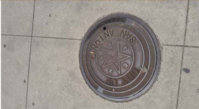
View of a Sanitary Sewer Manhole Cover, Potential Recharge Feature # S-1.
