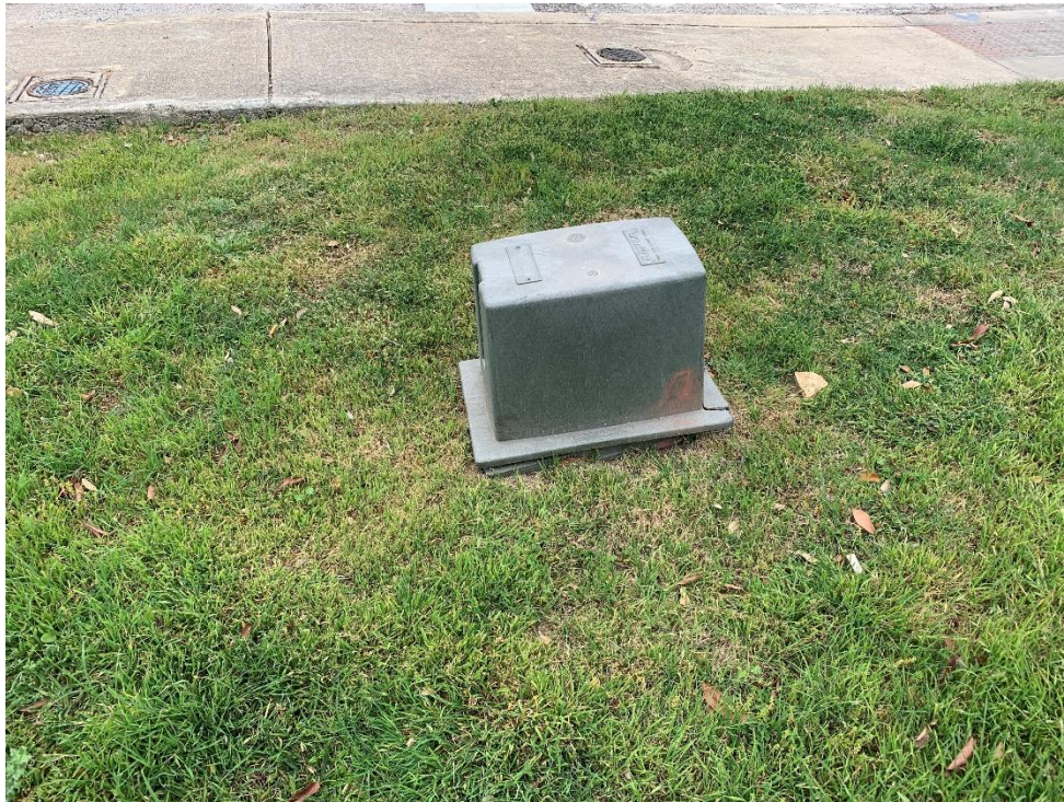
Photo #16: View of telecommunication box at the location of feature S-9.
