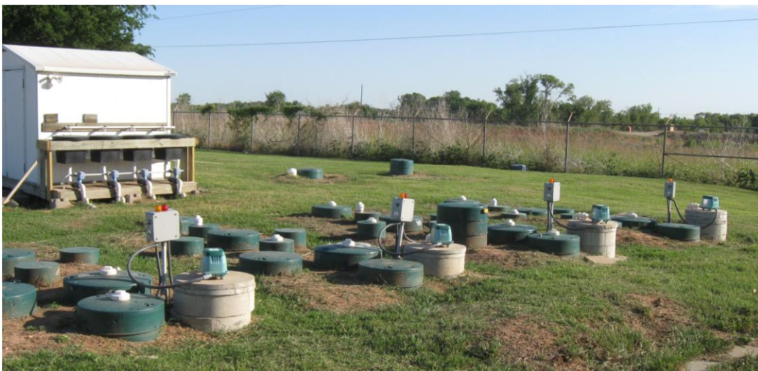
Figure 2. The enlarged new configuration showing the 4 aerobic systems with standard control panels and blowers in the foreground and the new, larger-capacity dosing buckets re-plumbed at the dosing shed in the background.
