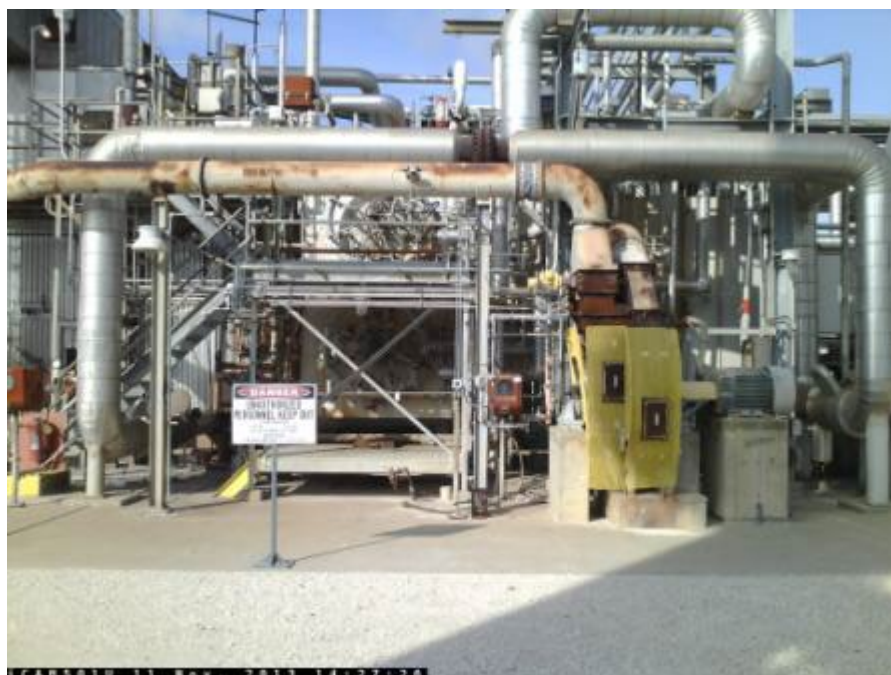
STEAM GENERATOR NO. 1 INJECTION AREA
