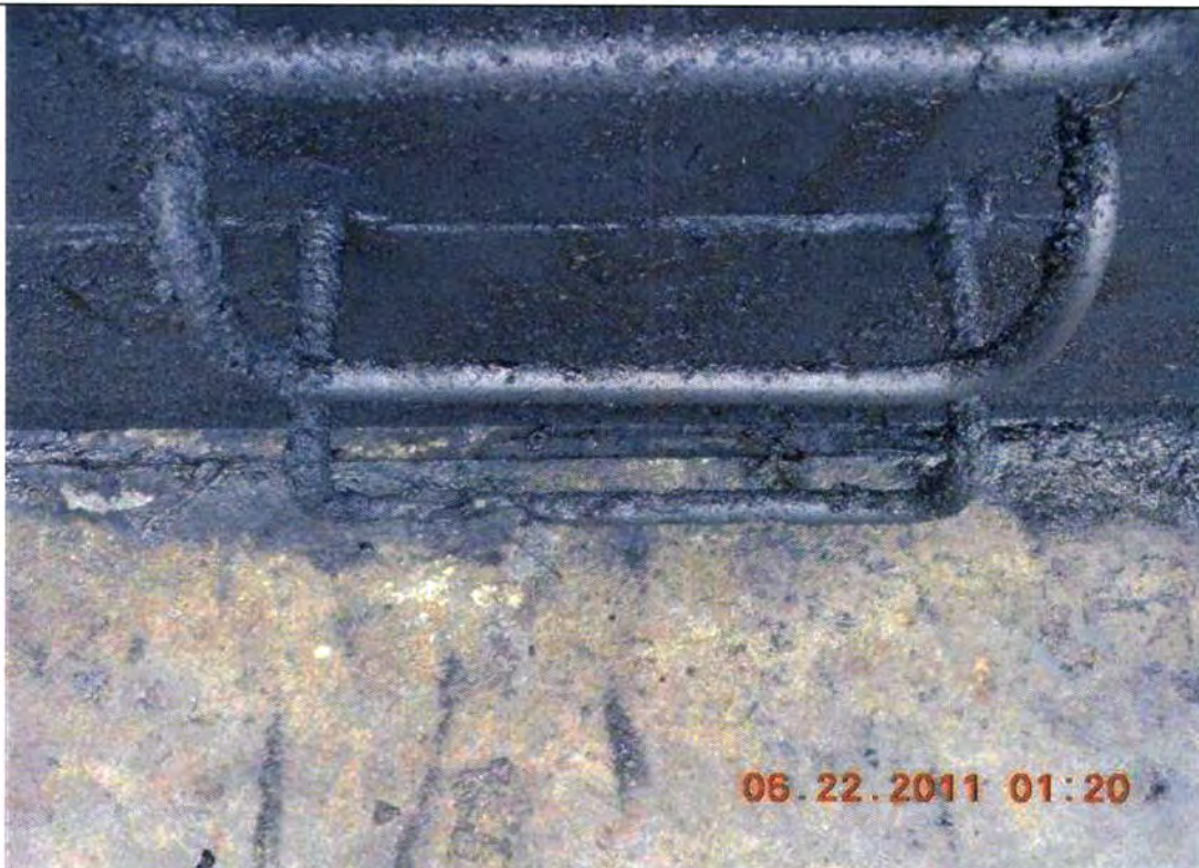
Photograph 8. View of corroded bottom ladder rung on the South interior Wall of the West Rain Basin.
