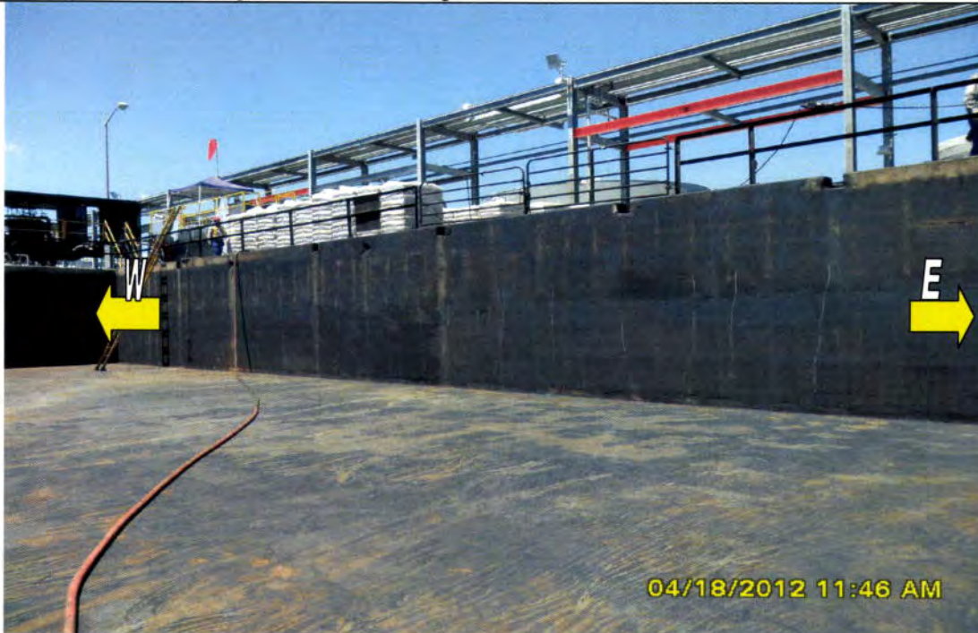
Photograph 2. View of North Wall from Southeast corner. Note Wall top scuppers and Typical crack propagation along the length of the Wall.
