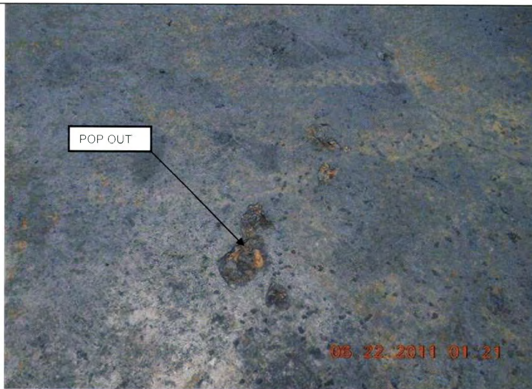
Photograph 10. View of aggregate "popout" on the Base Slab of the West Rain Basin.
