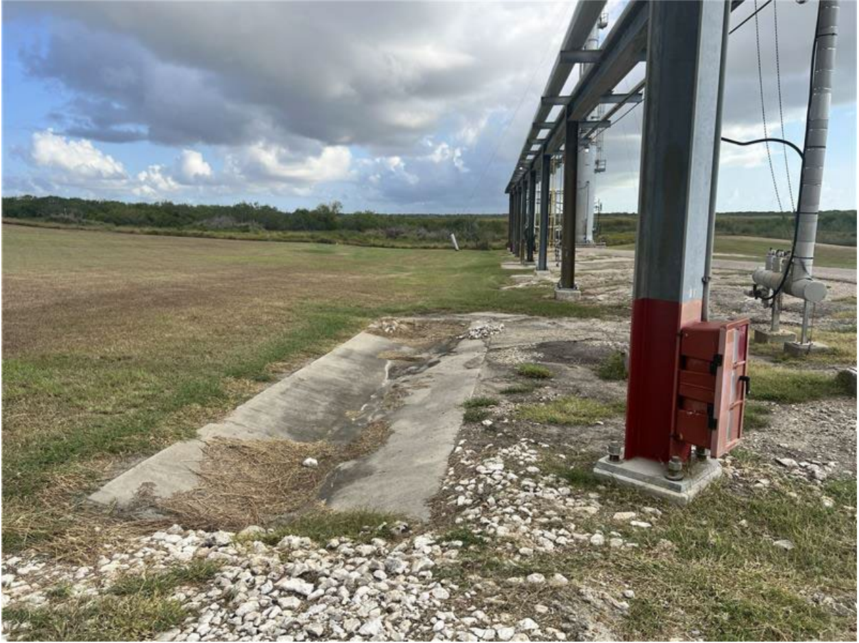
Fig 6. 003 Final discharge point facing southeast.
