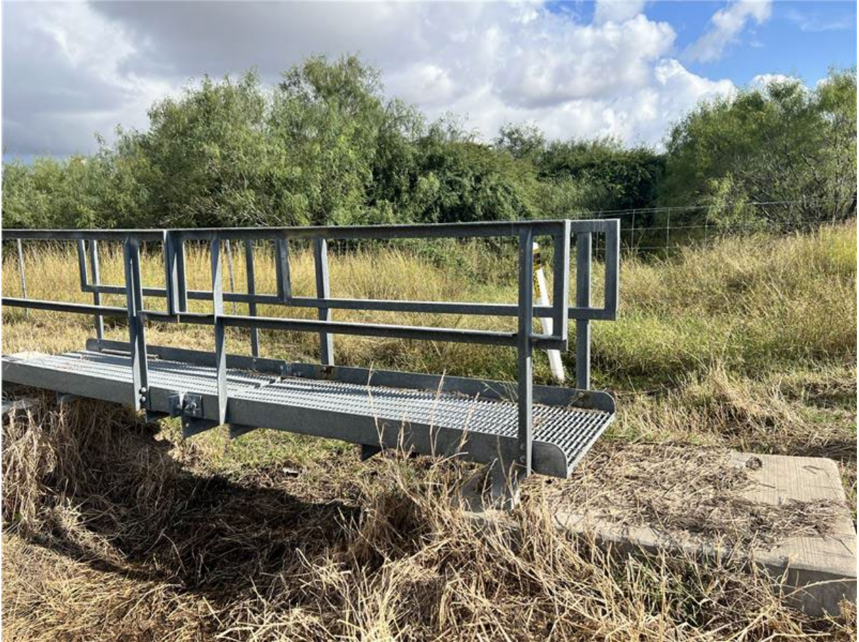
Fig 4. 002 Final discharge point facing southeast.
