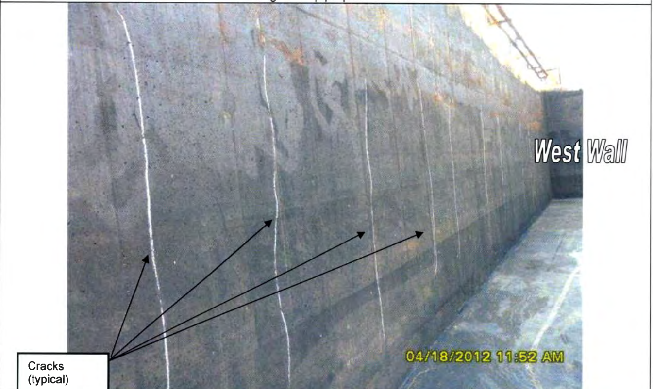
Photograph 6. View of South Wall from East corner. Note Typical crack propagation in East Rain Water Basin.
