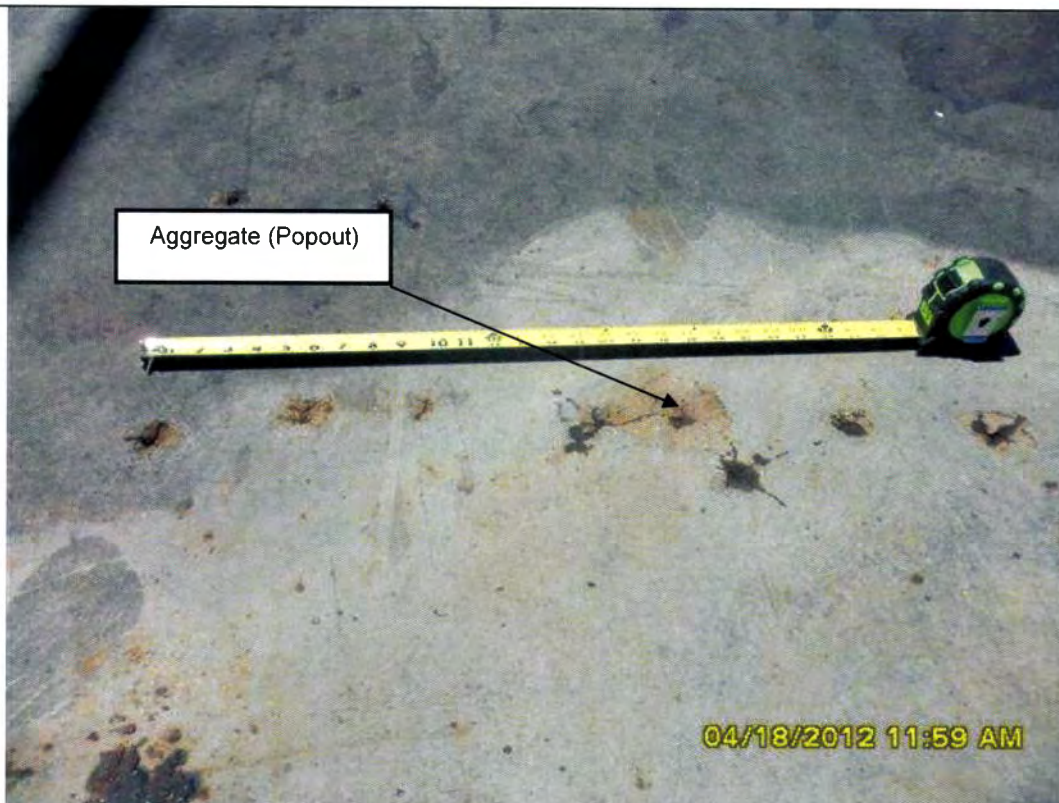
Photograph 10. View of Aggregate (Popout) on East Rain Water Basin Base Slab surface.
