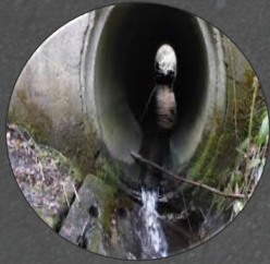
Storm Water Drainage Network (Production + Utility Area)
