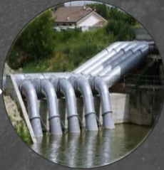
Storm Water Lift Station
