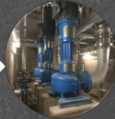
Storm Water Transfer Pump
