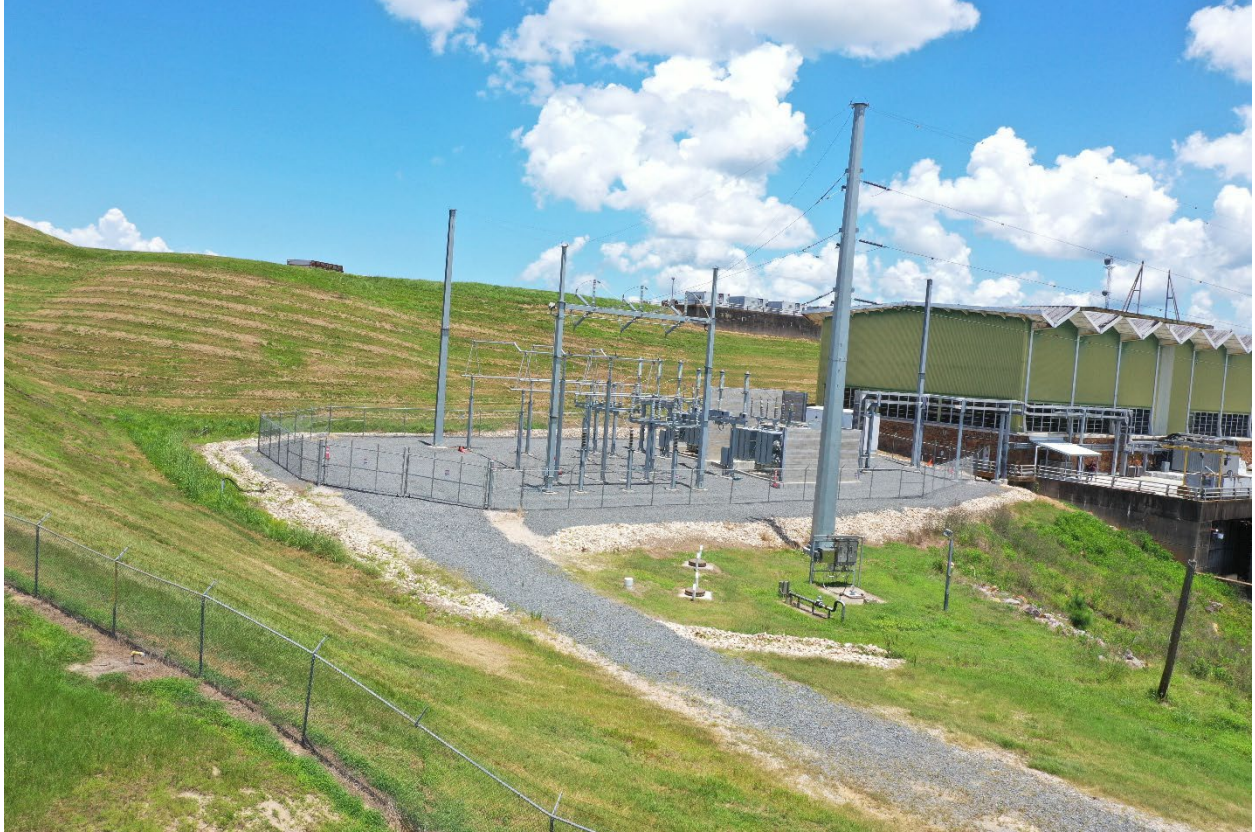
Photo 1: The new transformer yard.
