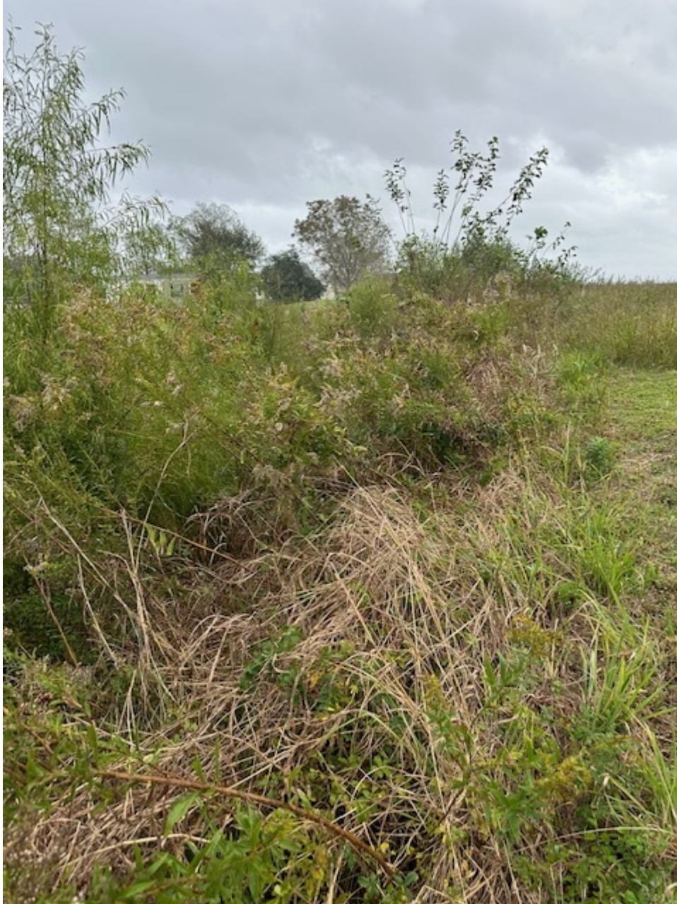
Photo 4 - Further downstream the channelized Cow Island Bayou is overgrown with vegetation.
