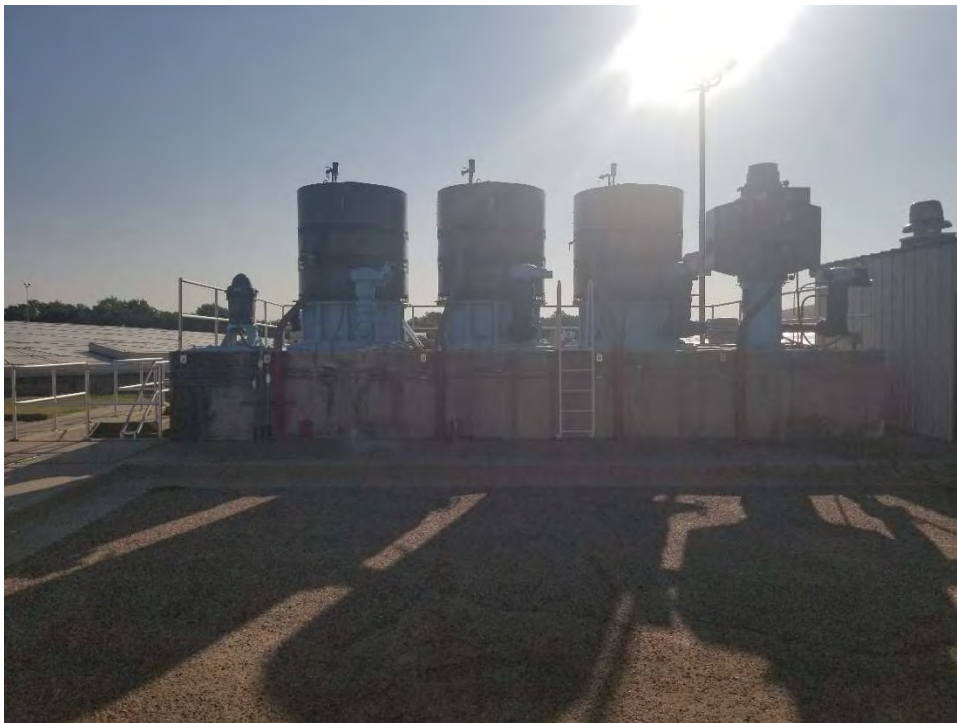
H.S. Pump Station, 1965
