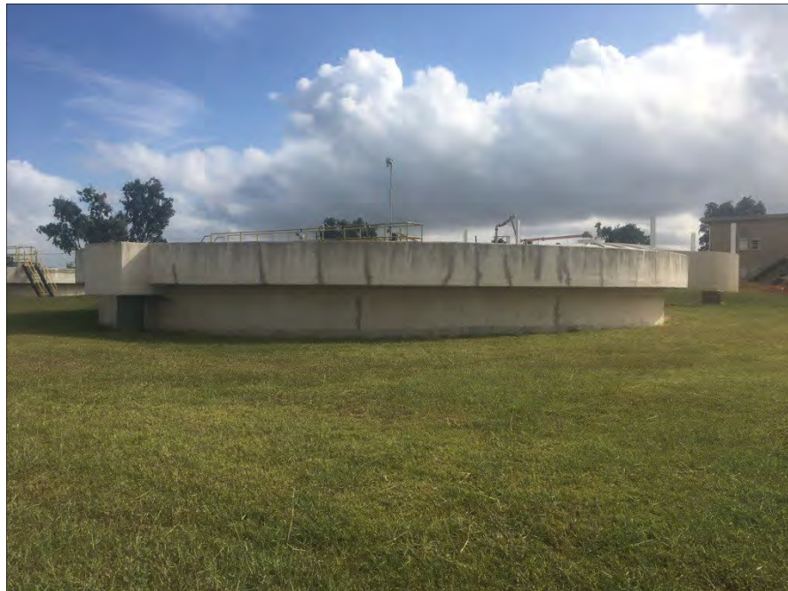
Photograph 2: Photograph of Primary Clarifier 2.
