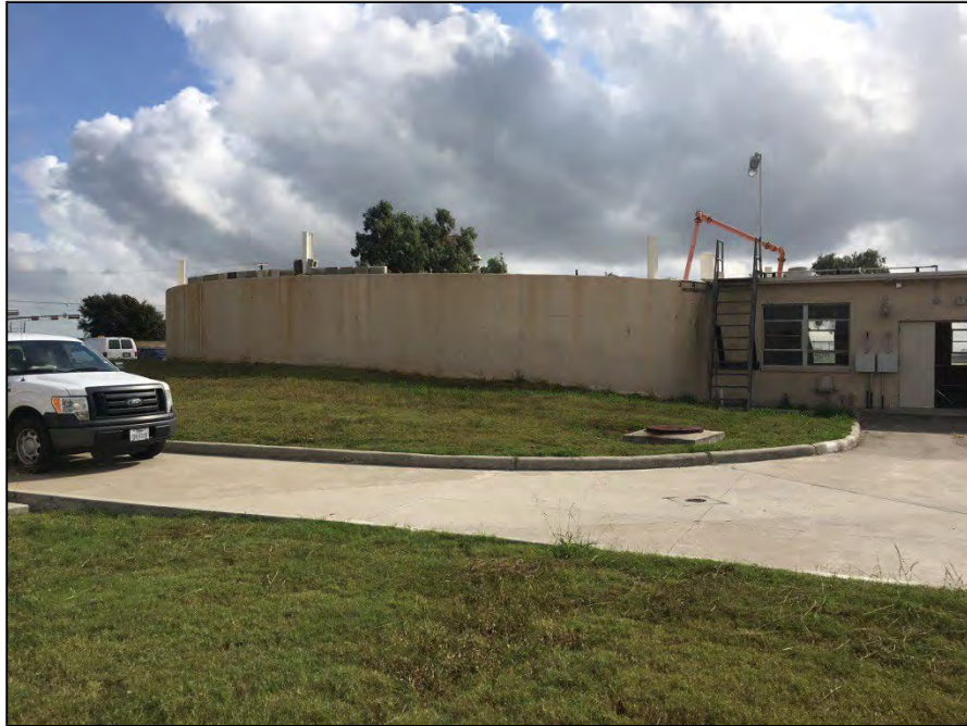
Photograph 5: Photograph of Sludge Digester 1.
