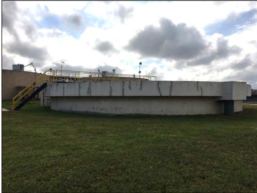
Photograph 3: Photograph of Primary Clarifier 3.
